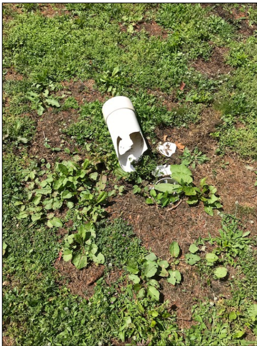
Broken Septic riser. Not bear damage
