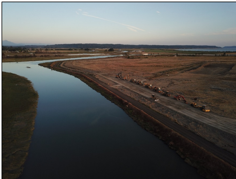
This photo shows the construction equipment parked for the night on top of the new wave protection berm, which will have a 0.7-mile long trail on top of it
