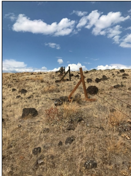
Boundary fence on Soda Springs Unit repaired with addition of five braces
