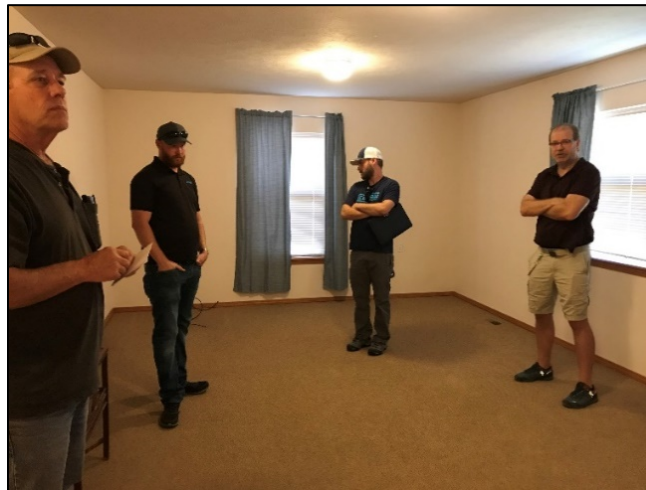
Left to right: Swanson Lakes Assistant Manager Mike Finch, two Cochran contractors, and Region 1 IT Specialist Mike Justice, inspecting residence to become the new office
