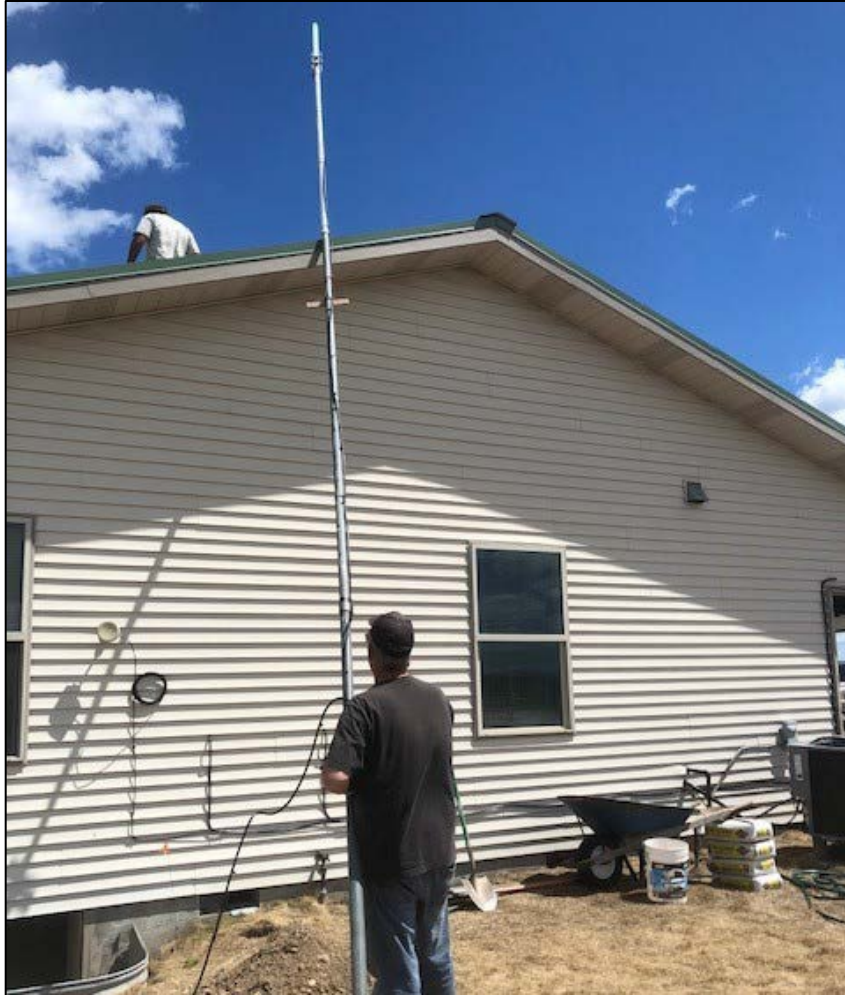
Swanson Lakes WLA Assistant Manager Mike Finch, supervising the installation of radio antenna at the new SL WLA office. The dead lawn will be replanted to native vegetation.
