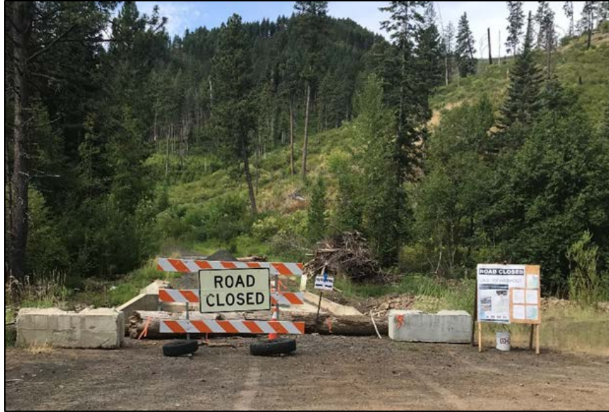
Road Closure now located at the Little Tucannon bridge washout
