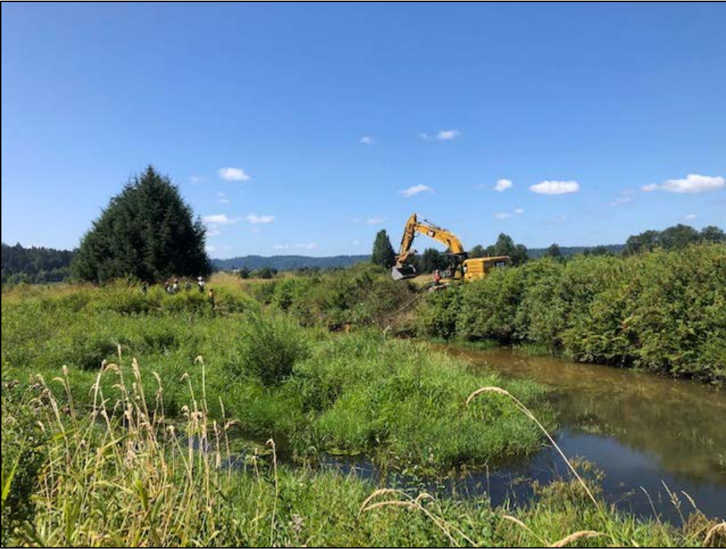
Construction equipment arrives at Cherry Valley Unit for the Drainage Improvement Project
