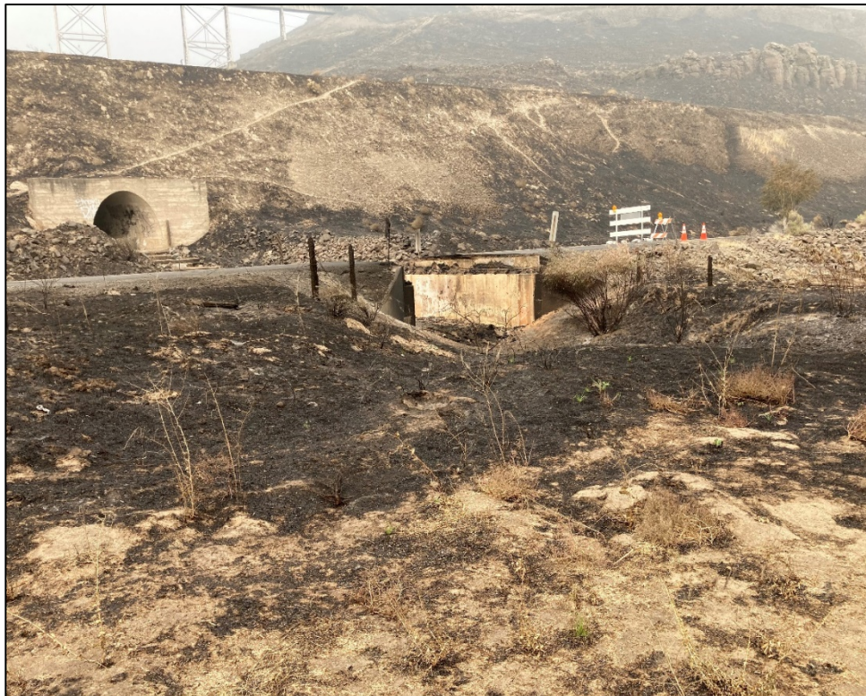
Burned bridge along the north shore of Snake River
