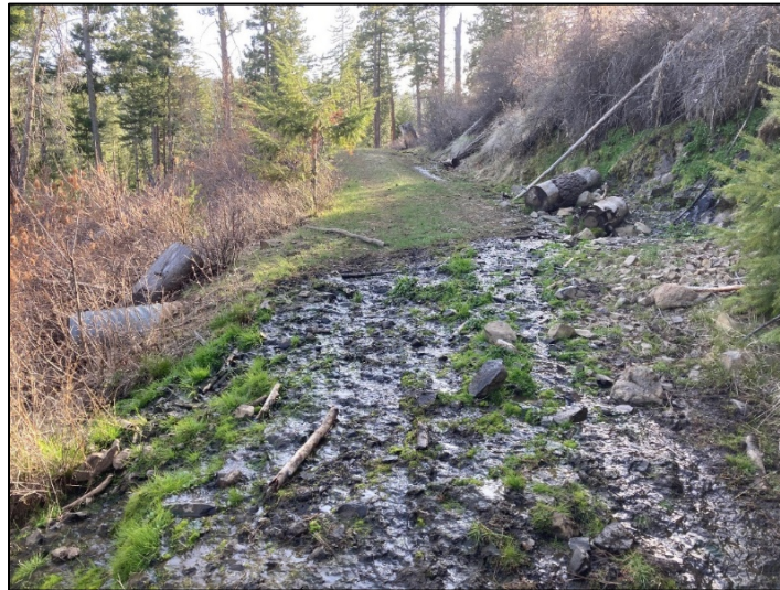
Plugged culvert on Colockum Wildlife Area road
