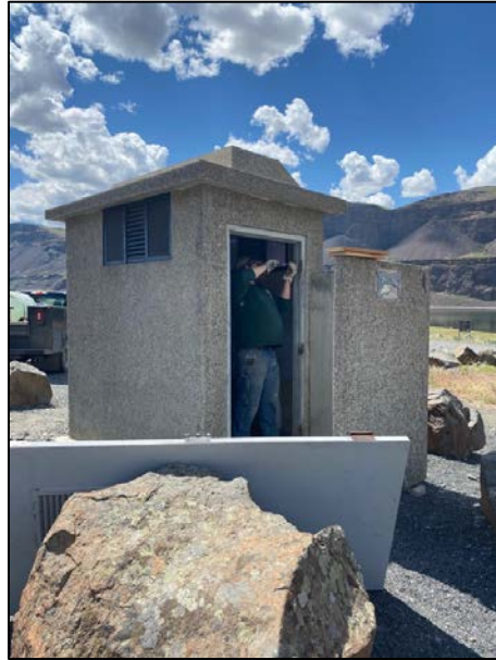
Steele installing the door frame at Sam Israel access site Lake Lenore – Photo by Harmon
