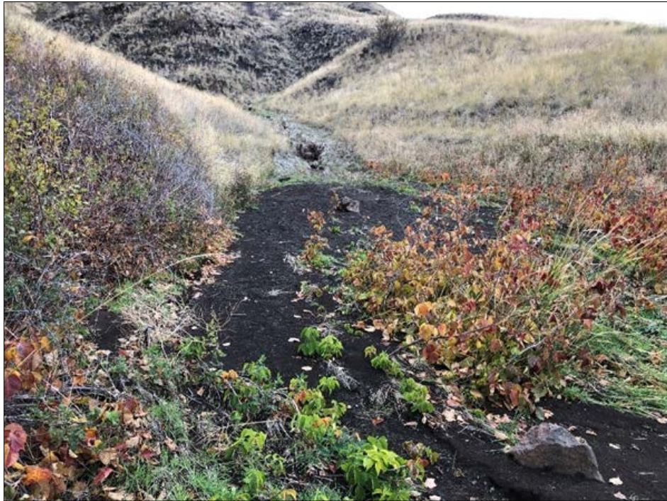
One of the numerous washouts covering the road near Birch Creek
