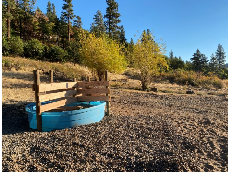
New stock tank and exclusion fencing around spring to protect wetland from domestic cattle
