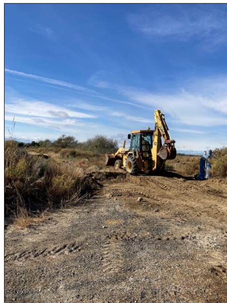
Assistant Manager Ferguson filling in the hole in the road using a backhoe
