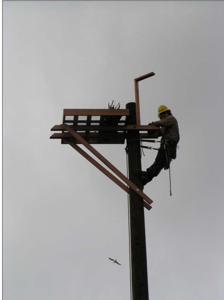
Almost done! A past Seattle Parks osprey platform effort that WDFW collaborated with due to opportunity (Burlington-Northern was willing to foot the bill) — Photo by C. Anderson
