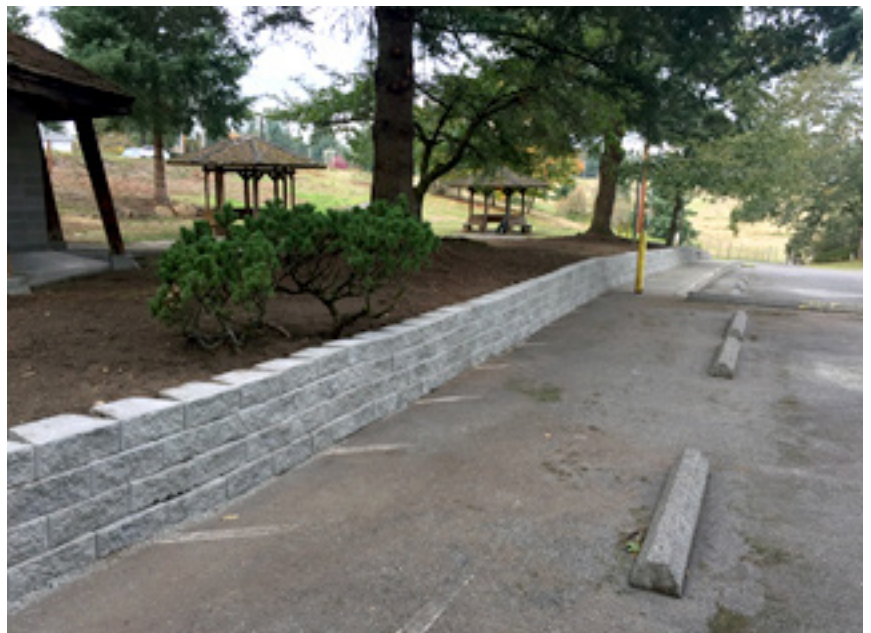
South Puget Sound Unit – renovated parking area completed by Clover Park Rotary. Photo by Alan Billingsley.
