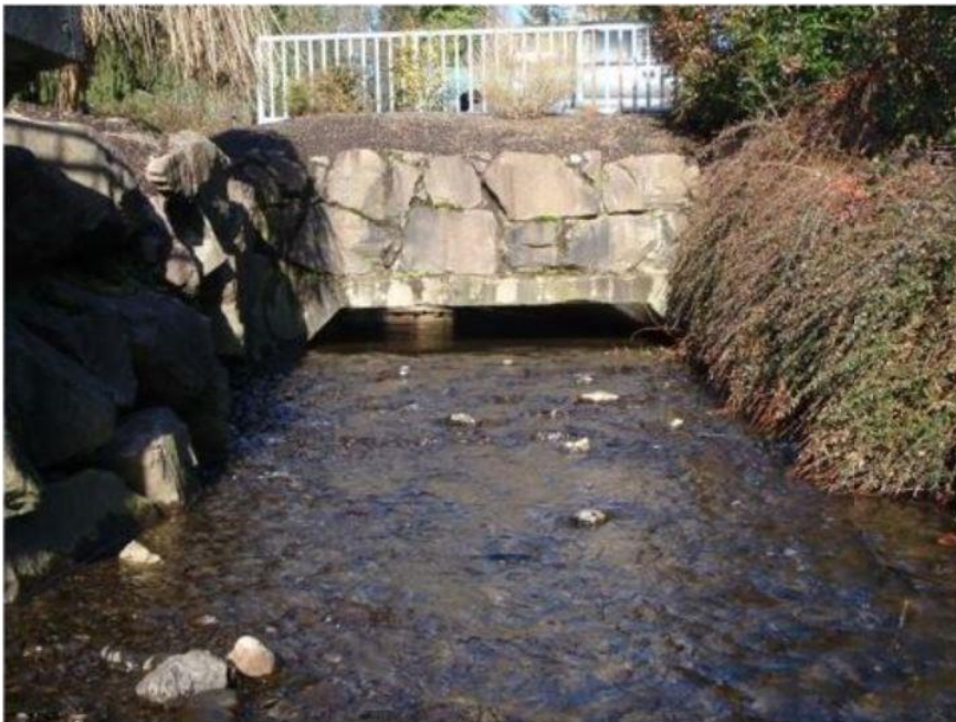
Figure 5. This is an example of a culvert that was assessed as fully passable more than ten years ago. In this case, the stream appears to have an active bedload and the clearance 11 years ago was minimal. It's possible that since 2009 this clearance has decreased enough for this site to be reassessed as a barrier. Site ID 930618. West Fork Kelsey Creek. WRIA 8.
