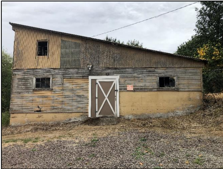
Deteriorating Cherry Valley barn ready for replacement
