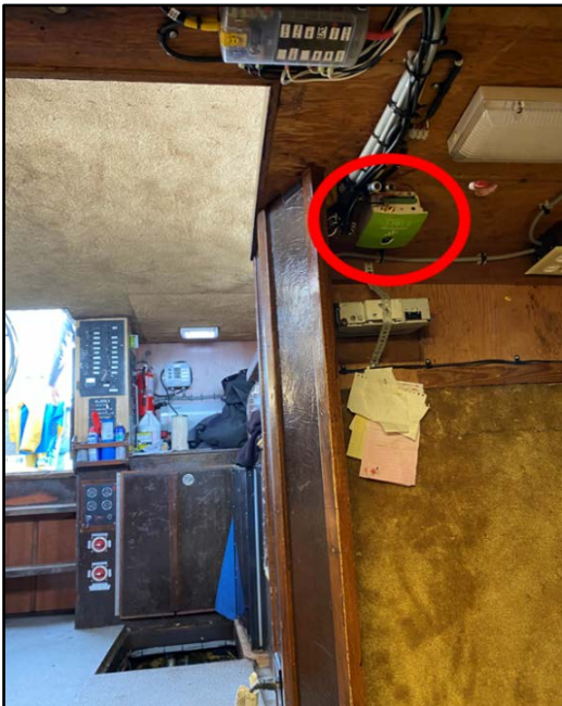
Figure 5. An installed LIME unit
