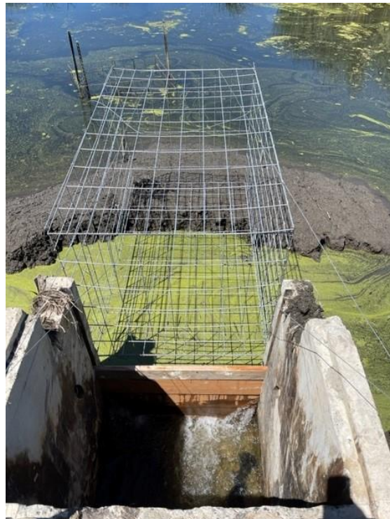
Beaver deceiver structure installed at the 7-acre pond outflow in the Mesa Lake Unit.
