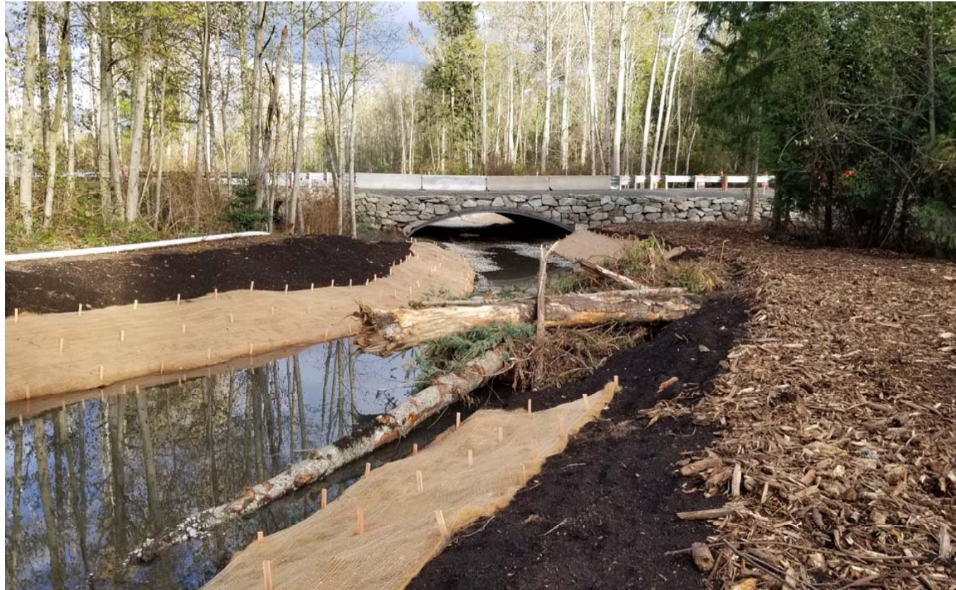
After: Bottomless Steel Plate Arch Culvert – 60 feet in length and 30 feet wide
