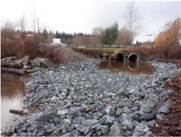
Before: Three Corrugated Metal Pipe Culverts – various lengths, and spans. Spall rock dumped throughout site.
