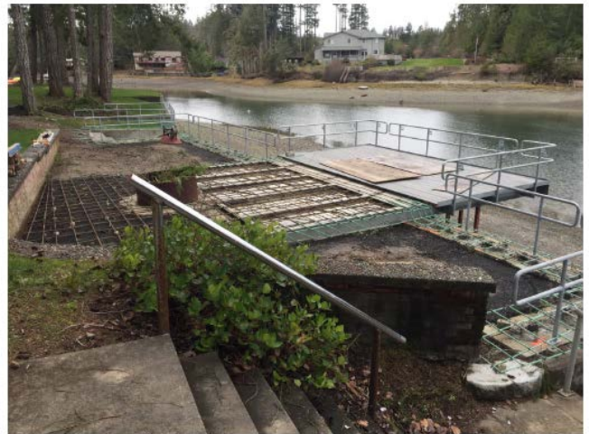
Photo taken March 2 nd , by Allison Cook. Shows upland view of construction work taking place on overwater structure. Decking surface over water is solid, with no functional grating.
