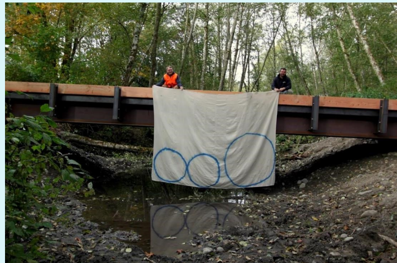
This new bridge across Upper Day Slough along the Skagit River, replaced the former culverts that blocked salmon migration (illustrated by blue circles).
