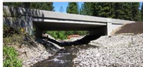
US 97 at Butler Creek after the $3.5 million barrier removal project was completed in April 2013.
