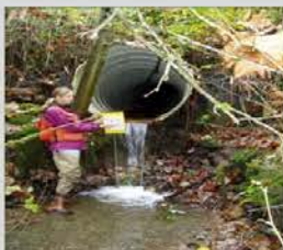
Excessive Water Surface Drop
