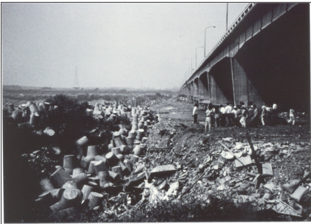
Figure 29. Undercutting and grade control efforts along the downstream side of the Kaoping Bridge over the Kaoping River, Taiwan, to control incision caused by massive gravel mining downstream (Photograph by Kondolf, October 1995).
