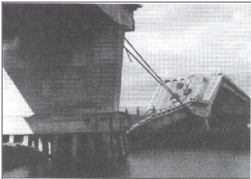
Figure 30. Failure of the Kaoping Bridge from gravel mining.
