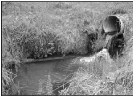
BPA Blocking Culvert
