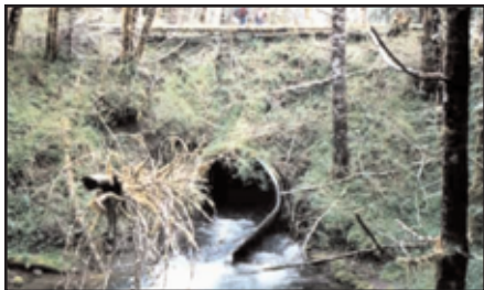
Bear Creek culvert, prior to removal, was a failing culvert with over 25' of fill.
