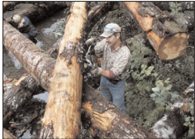
Dislocated fisherman cables instream ballasted log structures on North Fork Nooksack
