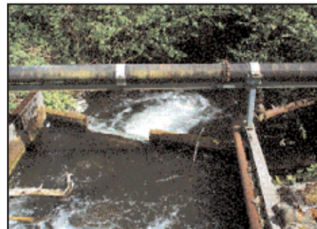
Stinger Creek blocking culvert
