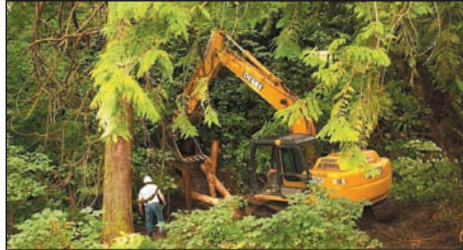
SFEG works with the Upper Skagit Tribe to install large woody debris in Red Creek.
