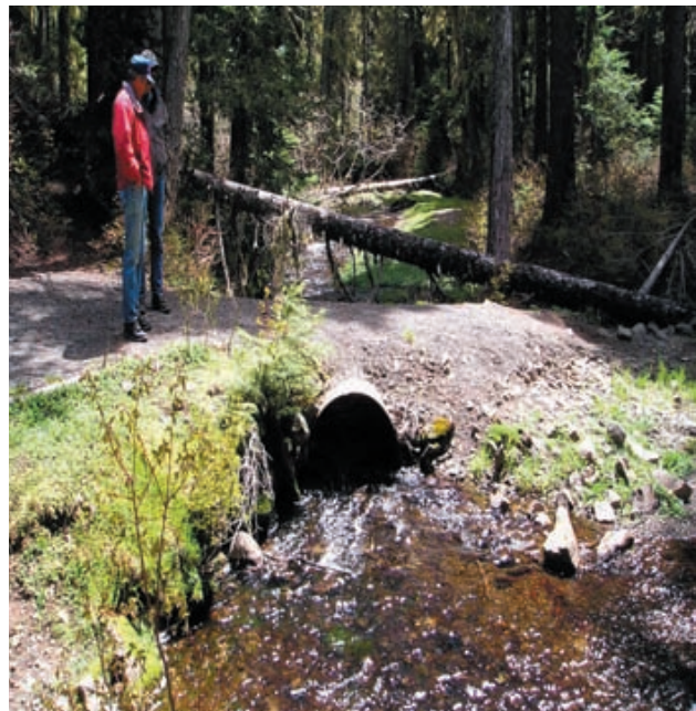
June 2005 - A culvert underneath the Pacific Crest Trail restricts stream flow at the White Pass South Trailhead
