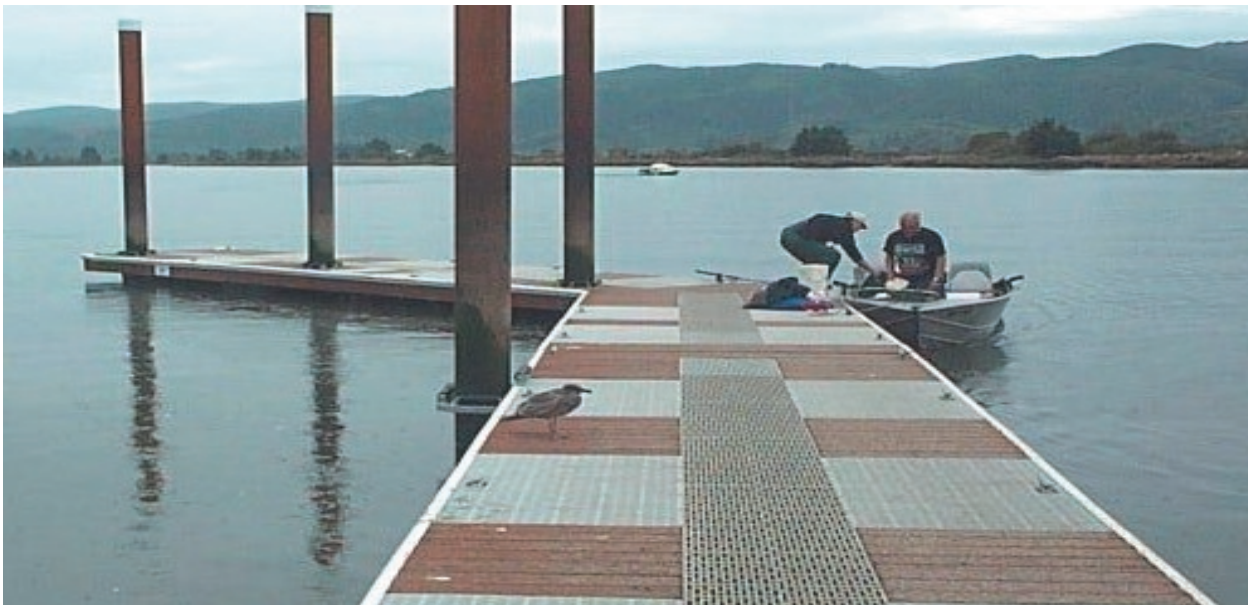
Community Outreach projects: Designed and installed additional 91 feet of floats/pilings for the City of South Bend Boat Launch.
