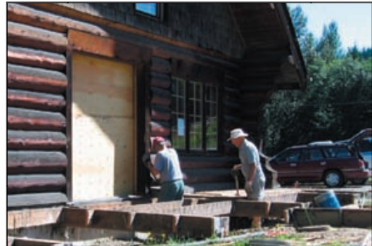
October 2005—Olympic Discovery Nature Center work party. Volunteers work together to remove deck material.
