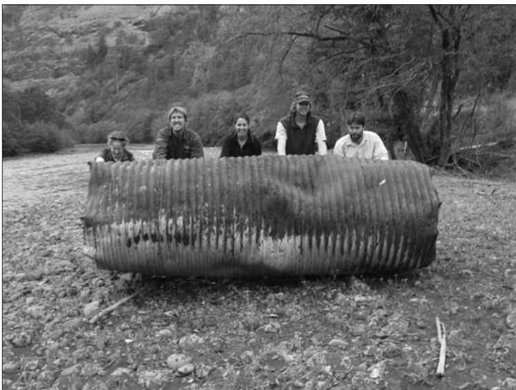
Crew members roll this culvert to higher ground after removing it by hand from the Klickitat River. - October 2006
