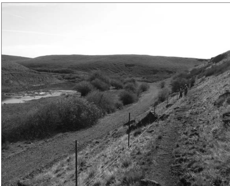
Crew members constructing a livestock exclusion fence on Swale Creek, a tributary to the Klickitat River. - April, 2007
