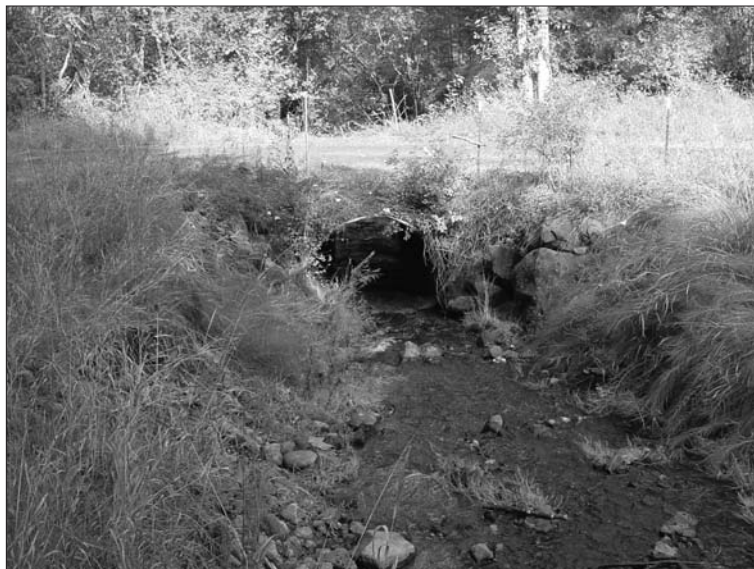
Before – Undersized culvert in Jim Creek.
