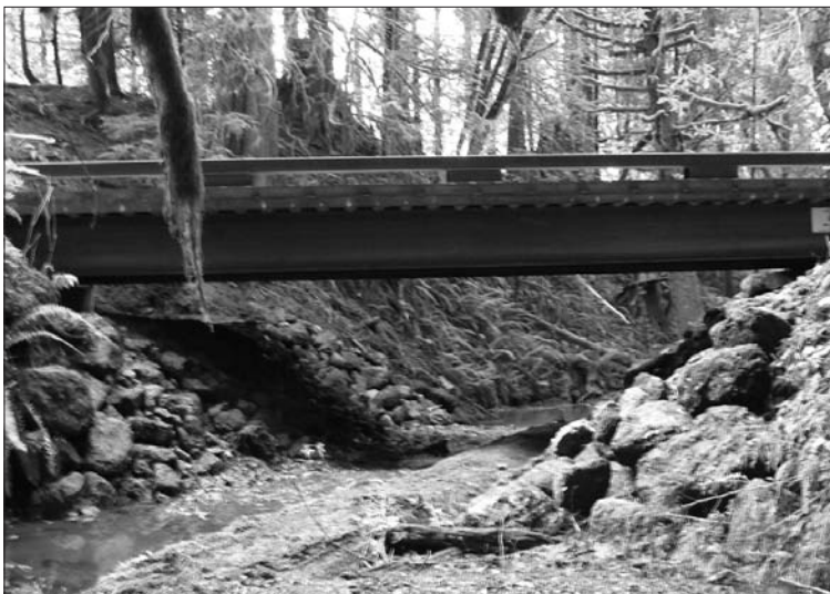
The Tosland Project addressed three parallel culverts that were 33% passable with a 40 ft. long, 14 ft. wide bridge (shown above), opening 1.3 miles of habitat for Coho, Cutthroat, Searun Cutthroat, and Steelhead at a cost of $101,000.
