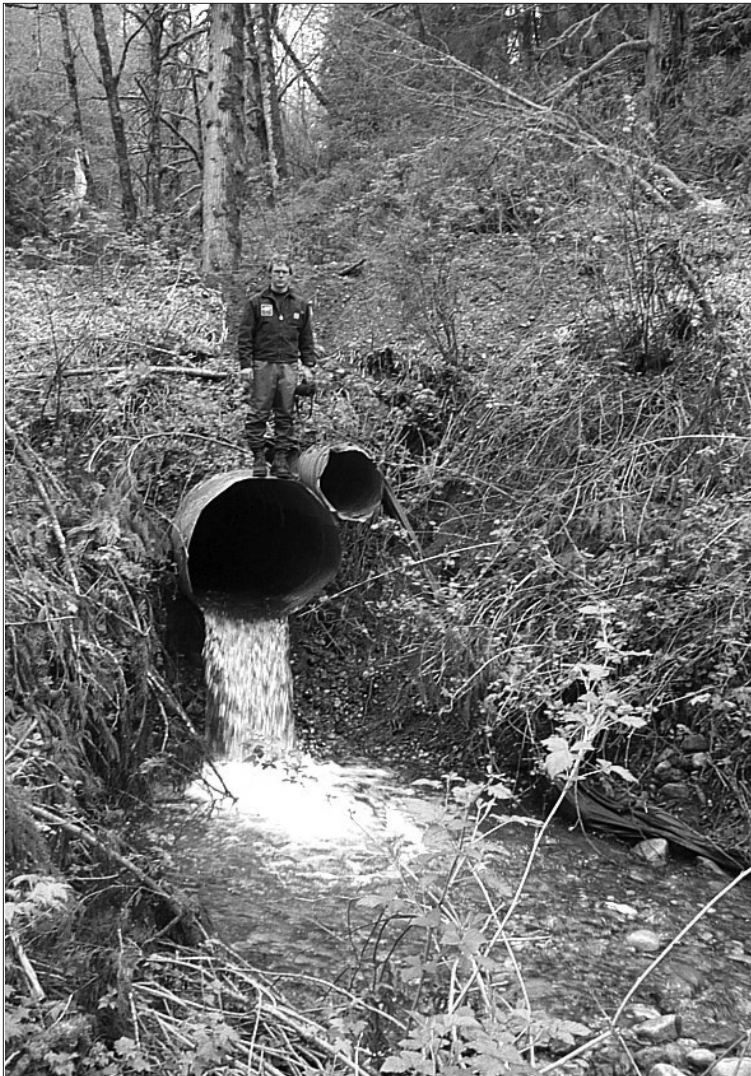
Before picture of perched culvert at Parson’s Creek.
