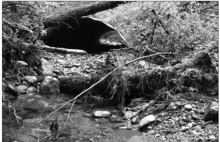
After picture of new culvert at Parson’s Creek crossing to improve salmon and steelhead access to upper watershed habitat.
