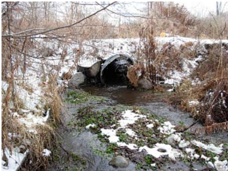
Antoine Creek, undersized culvert
