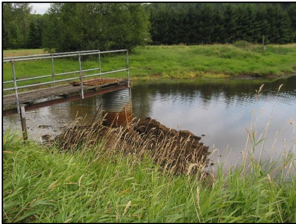
Failed Mossyrock Riser Pond #1
