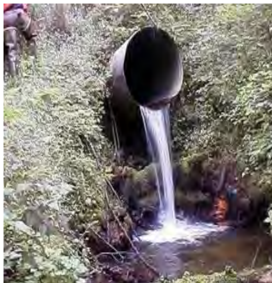
Figure 3-10. Drainage culvert projects are one type of activity contained in the HPMS database.
