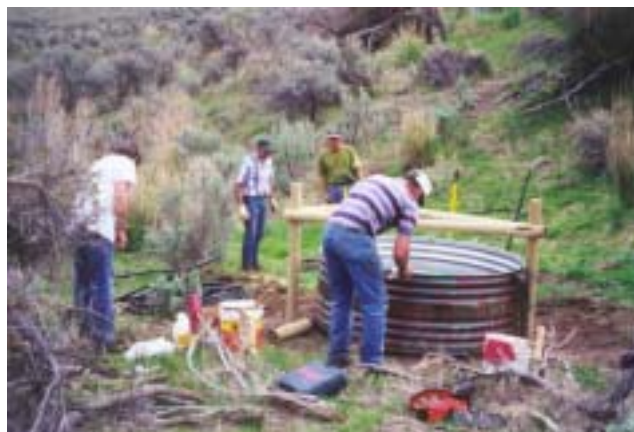
Volunteers from the Wenatchee Sportsman’s Association construct a water tank in the Collin Springs area to benefit elk, deer, bighorn sheep and other wildlife.
