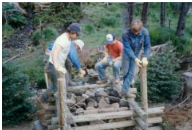
Members of the Washington Conservation Corps build a rock jack fence on a WDFW Wildlife Area in eastern Washington.
