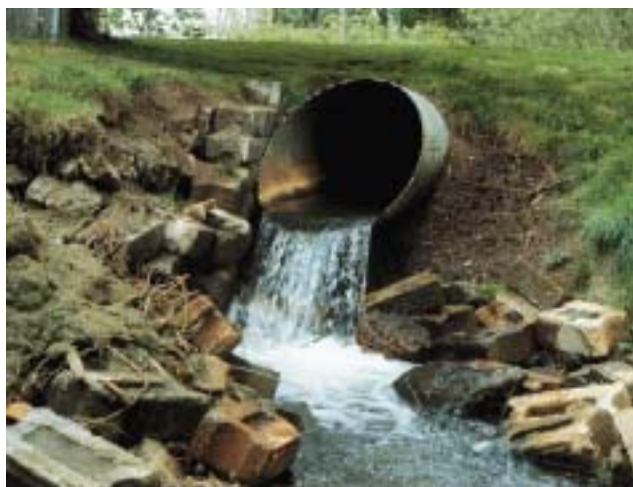
"Hanging culverts" like this one present a major barrier to fish passage and are being replaced through a partnership with the Washington Department of Transportation.
