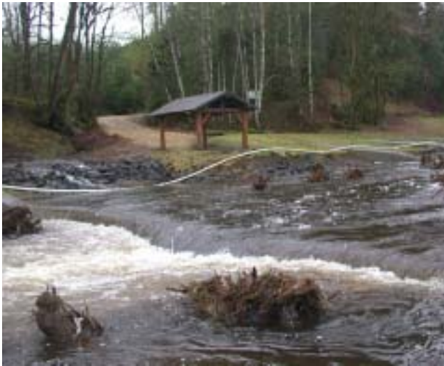
Weirs installed at Goldsborough Creek create a gentle cascade where an aging wooden dam formerly presented a formidable barrier to migrating fish. Project partners included WDFW, the Army Corps of Engineers and Simpson Timber.
