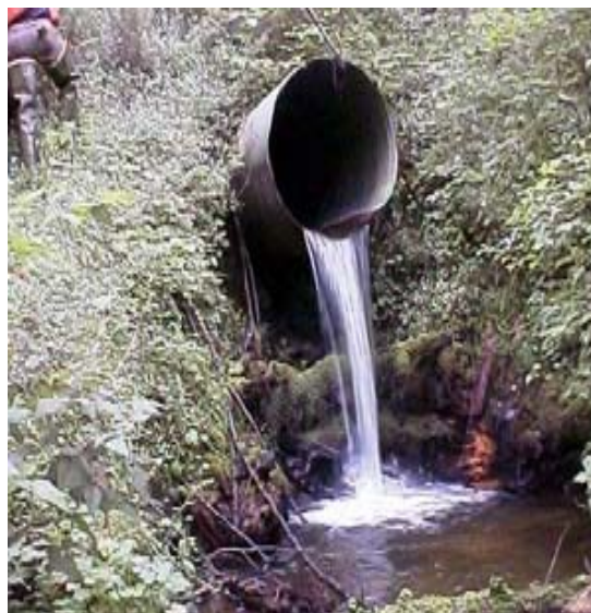
Figure 3-6. Drainage culvert projects are one type of activity contained in the HPMS database.
