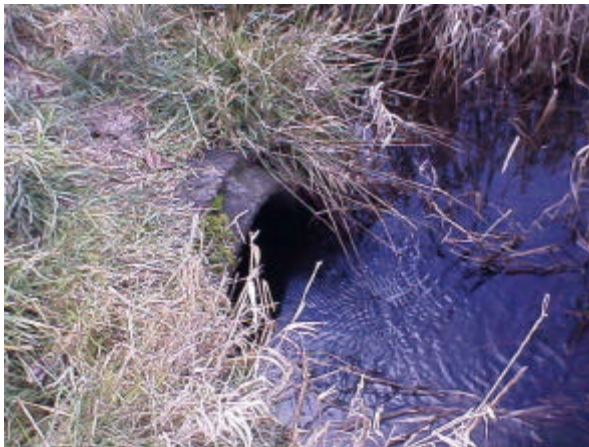
Photo 11. Site 980932, Unnamed tributary to Unnamed tributary to Cowlitz River. Having 1% slope with no streambed material throughout the inside of the culvert, this site is considered a partial barrier to fish passage.
