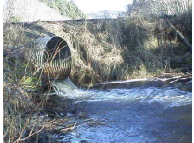
Photo 30. Site 981077, Simmons Creek (26.0631) tributary to Riffe Lake. With large headwater ponds directly upstream, this total barrier culvert blocks fish access to more than 6,300 square meters of quality rearing habitat.
