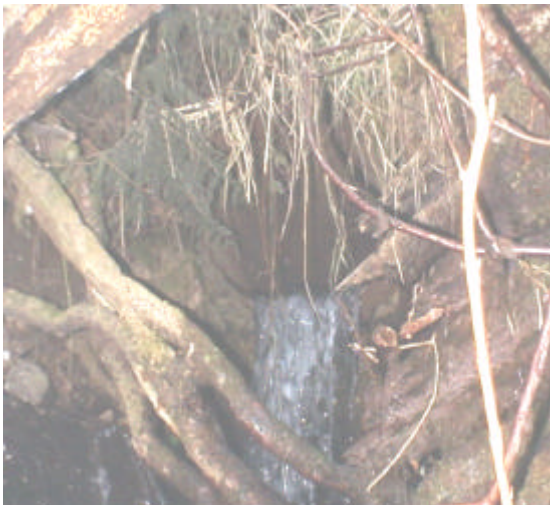
Photo 27. Site 980796, Unnamed tributary to Unnamed tributary (26.0641) to Shelton Creek. With a 1.5 meter outfall drop and a 3% slope, this culvert is a total barrier to fish passage.
