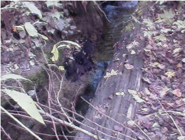
Photo 19. Site 981304, Unnamed tributary to Shelton Creek. The obstructed stream flow caused by this timber made culvert is cutting at the right bank. This is a good view of the large timbers placed parallel within the channel. This site is a partial barrier to fish passage.
