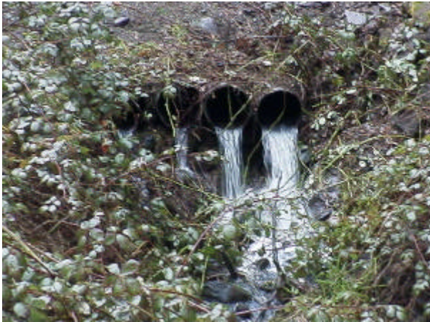
Photo 37. Site 981103, Mayfield North, Unnamed tributary to Mayfield Lake. This culvert crossing is less than 25 meters upstream of the lake. Correcting fish passage of this total barrier will allow anadromous and resident fishes upstream access to approximately 1,046 linear meters of stream.
