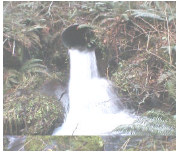
Photo 28. Site 980729, Unnamed tributary to Unnamed tributary (26.0641) to Shelton Creek. Because this culvert is undersized and has a 1.6 meter outfall drop and a 5% slope, it is a total barrier to fish passage.
