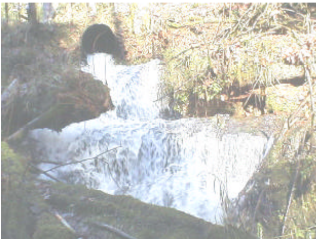
Photo 31. Site 980737, Unnamed tributary to Riffe Lake. While this high gradient stream possesses difficult obstacles for fish movement, the culvert is considered a fish passage barrier due to inadequate size and a 6% slope. There are three additional barrier culverts downstream on DNR property.
