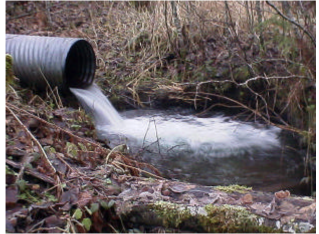
Photo 26. Site 980793, Unnamed tributary to Unnamed tributary (26.0641) to Shelton Creek. This photo illustrates how the installation of an undersized culvert can create obstacles that inhibit fish passage. The velocity and outfall drop impedes fish passage and this culvert is a total barrier.
