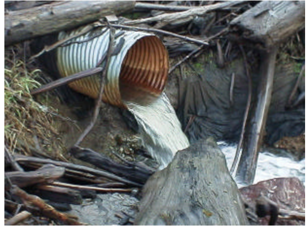
Photo 6. Site 980854 continued. Outlet of pond drains directly into Rainey Creek. No streams feed the pond and only rearing habitat exists upstream. This site is considered a total barrier to fish passage.
