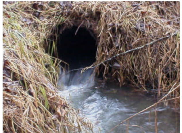
Photo 8. Site 980852, Unnamed tributary to Steffen Creek. Because this culvert is undersized and has 5 % slope, high velocities create a total barrier to fish passage.
