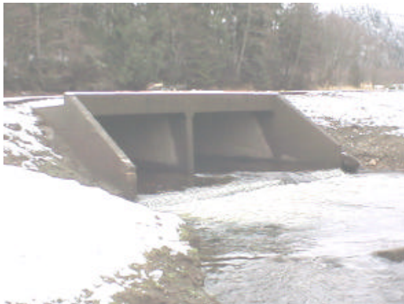
Photo 35. Site 980921, Swofford Pond outlet to Riffe Lake. This partial barrier culvert becomes backwatered and passable when the stage of Riffe Lake is raised.
