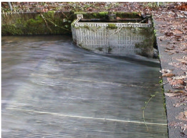
Photo 3. Site 980911 continued. Side view of this site shows the hatchery rack and the gravity diversion intake on the left bank. Because the diversion is no longer in use, the features should be removed.
