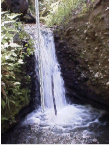
Photo 41. Site 981233, Riffe South, Unnamed tributary to Riffe Lake. This barrier outfall drop is likely the result of the undersized culvert that washed out sometime in the past.
