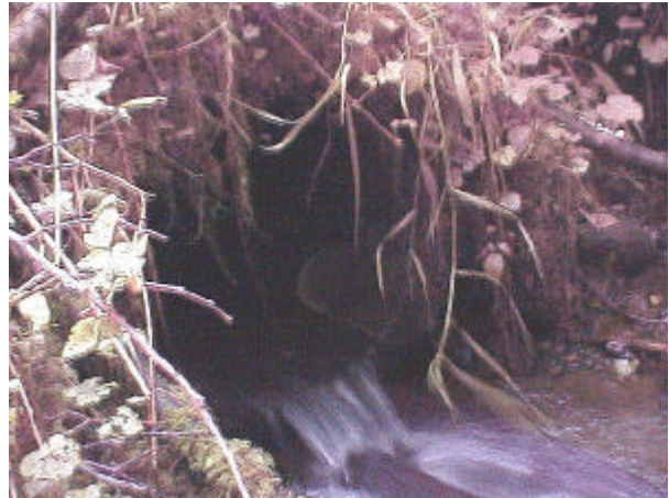
Photo 38. Site 981273, Riffe North, Unnamed tributary to Riffe Lake. Located under an abandoned black top road, this partial barrier culvert is undersized and has a 2% slope.
