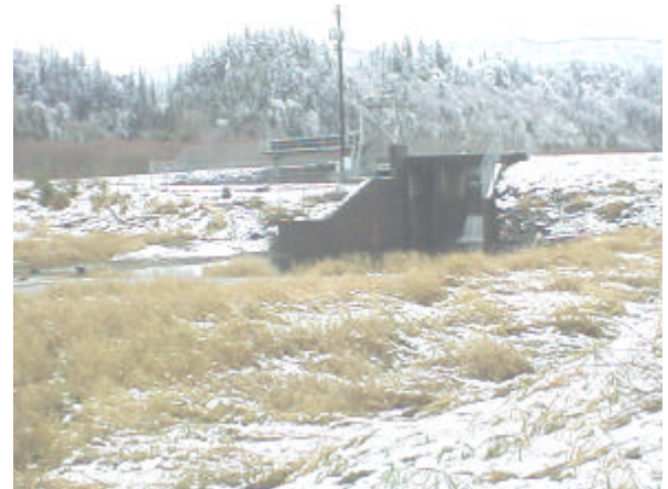
Photo 36. Site 980920, Swofford Pond (Sulphur Creek, 26.0628). Distant view of dam and lake outlet structure. Although this barrier would require repair to pass salmonids, the upstream habitat is more suitable for warm water fish. The current warm water fishery is popular and likely the best choice for this small sub-basin watershed.
