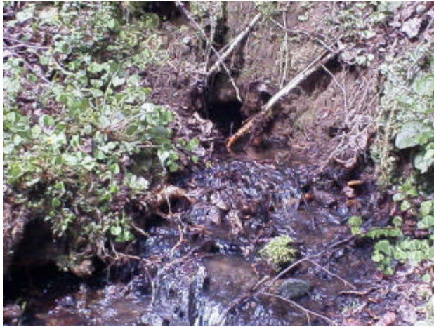
Photo 25. Site 981207. Unnamed tributary to Unnamed tributary (26.0641) to Shelton Creek. This timber-made crossing appears to be mostly clogged and the flow constricted. This site was evaluated as a partial barrier at the time of the survey.
