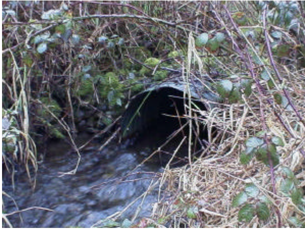
Photo 9. Site 981159, Unnamed tributary to Cowlitz River. This culvert is undersized and set at greater than 1 % slope, creating high velocity flows and a total barrier to fish passage.
