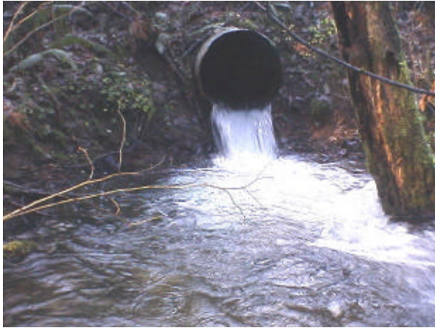
Photo 21. Site 980701, Unnamed tributary to Shelton Creek. This photo depicts two reasons why this culvert is a total fish passage barrier: (1) excessive velocity created by an undersized pipe with a 3% slope, and (2) outfall drop greater than 0.30 meter.
