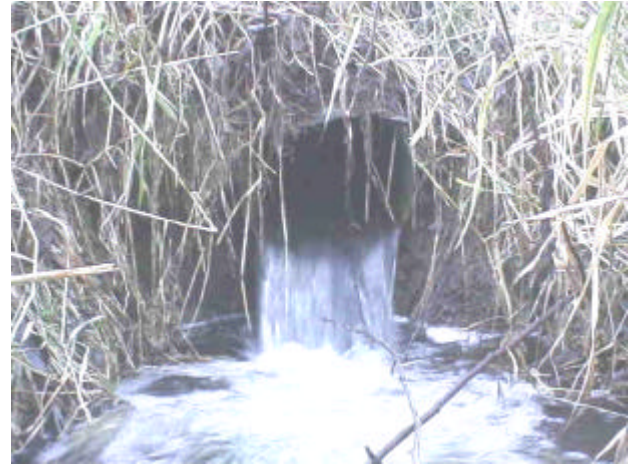
Photo 34. Site 980747, Unnamed tributary to Unnamed tributary to Riffe Lake. This photo illustrates an undersized culvert with slope greater than 1% and severe outfall drop creating a barrier to juvenile and adult salmonids.
