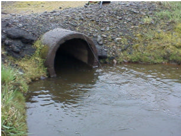
Photo 7. Site 981177, Unnamed tributary to Steffen Creek. Having greater than 1% slope and no streambed material throughout the culvert, this culvert is considered a partial barrier to fish passage due to velocity. This site becomes inundated by Riffe Lake during the summer recreation season.
