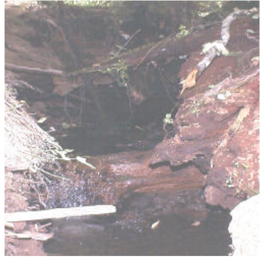
Photo 18. Site 981296, Shelton Creek (26.0640) tributary to Riffe Lake. This timber-made culvert has failed. The outfall drop impedes fish passage during low flow periods.
