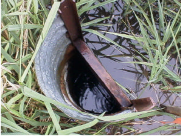
Photo 13. Site 981172, Unnamed tributary to Unnamed tributary to Cowlitz River. Created for waterfowl enhancement, this dam with a water control structure is a complete barrier to fish passage.
