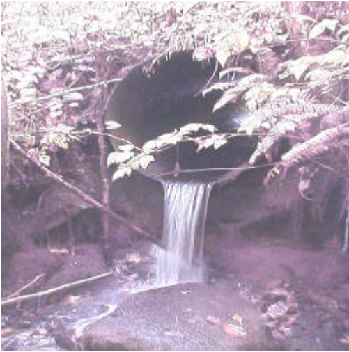
Photo 17. Site 981294, Shelton Creek (26.0640) tributary to Riffe Lake. This culvert is a total barrier due to the outfall drop and no plunge pool. Because the culvert is perched and undersize, streambed material passes through rather than settling out.
