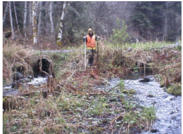
Photo 16. Site 980761, Shelton Creek (26.0640) tributary to Riffe Lake. This double culvert crossing is undersized and a partial barrier to fish passage. The right bank pipe is impassible due to velocity. The left bank pipe becomes a velocity barrier during high flows.
