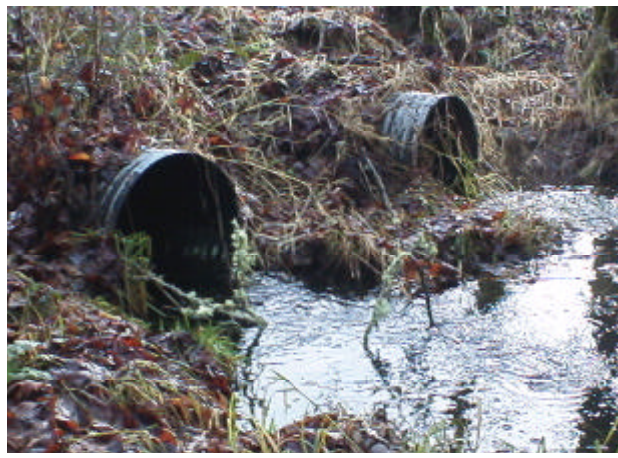
Photo 4. Site 980918, Alexander Creek (26.0528) tributary to Blue Creek. Both culverts at this site have a 3% slope and lack streambed material throughout the inside of the culverts. This site is considered a partial barrier to fish passage due to velocity.
