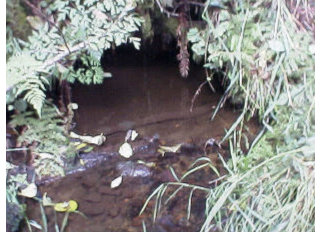
Photo 22. Site 981297, Unnamed tributary to Shelton Creek. Several sections of this timber made culvert have failed. Flow through this structure is obstructed, which partially blocks fish passage.
