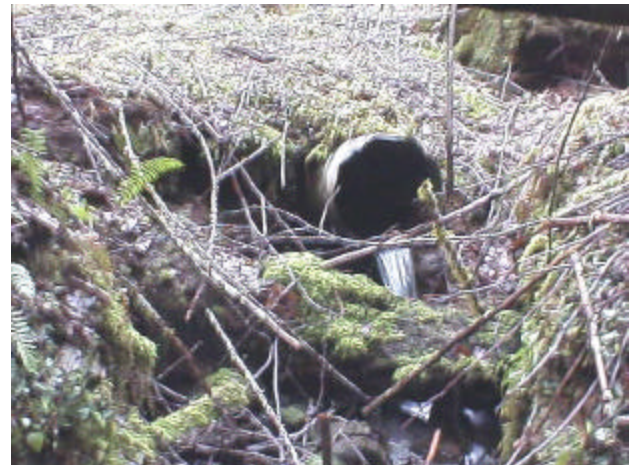
Photo 24. Site 981136, Unnamed tributary to Unnamed tributary (26.0641) to Shelton Creek. A 0.46 meter corrugated steel pipe was added to this clogged timber made culvert crossing. The road prism atop this crossing has failed and is no longer drivable. This site is a total barrier to fish passage.
