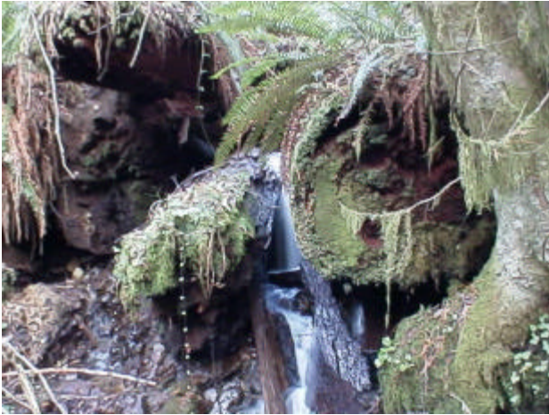
Photo 29. Site 980812. Unnamed tributary to Unnamed tributary (26.0641) to Shelton Creek. Flow and fish passage are completely obstructed through this timber made culvert.
