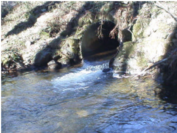
Photo 23. Site 980817, Unnamed tributary (26.0641) to Shelton Creek. This culvert is undersized with greater than 1% slope, posing a velocity barrier to adult and juvenile fish passage, depending on flow conditions.
