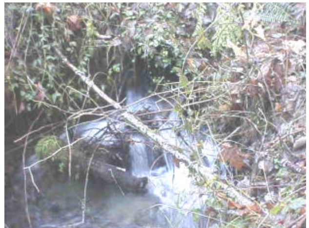
Photo 32. Site 980750, Unnamed tributary to Unnamed tributary to Riffe Lake. Several reasons why this culvert is a total barrier to fish passage include: 2% slope, 0.30 meter outfall drop, and inadequate pipe size constricting the flow causing high velocities.
