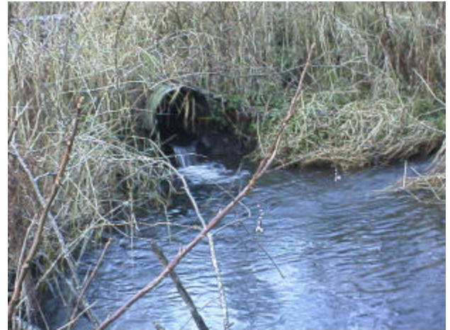
Photo 20. Site 980779, Unnamed tributary to Shelton Creek. Although this site has an overflow pipe, the culvert is undersized and has a 5% slope. This culvert is a total barrier to fish passage.
