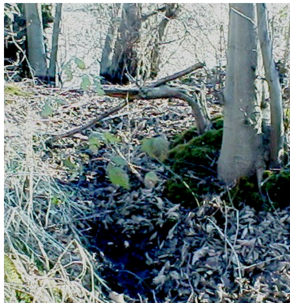
Figure 13. Site 981796. An earthen dam with a spillway. Pond water spills over the top of the earth dam into an overflow channel. Rarely, if ever, is there enough flow for fish to use the channel. The pond has 1,407 square meters of potential rearing habitat. The PI for this total barrier is 3.61.
