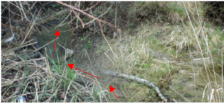
Figure 26. Site 981814 at Claypit Pond. This earthen dam has an overflow channel that empties into Tennant Creek. The photo shows the dam spillway and the direction of the overflow channel. At the outlet of the channel is a culvert that carries some flow but has no apparent function. Claypit pond provides 9,033 square meters of potential rearing habitat. The PI value is 15.33.
