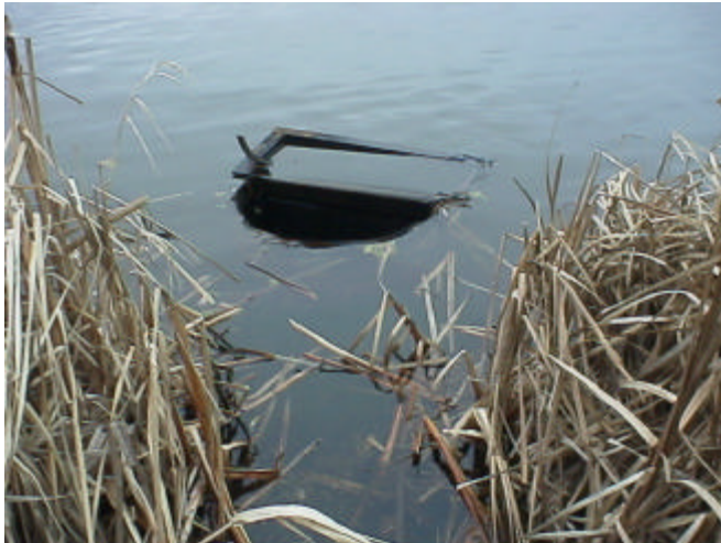
Figure 8. Site 981785 consists of an earthen dam with a standpipe. This total barrier to fish passage blocks access to 0.50 km (0.31 miles) of stream containing 6,081 square meters of rearing habitat. The PI value for this barrier is 18.33.
