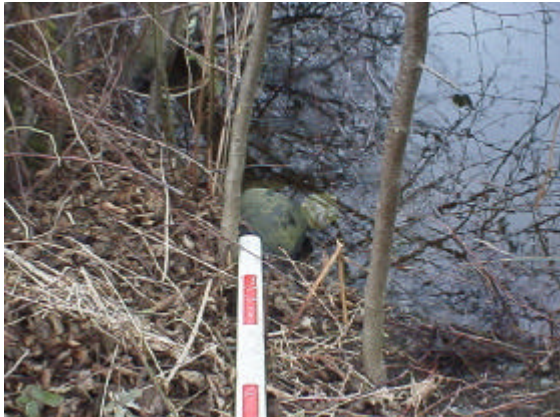
Figure 10. Site 981781. An earthen dam with a 0.21 meter overflow culvert creates a small pond. The pond has 1,219 square meters of potential rearing habitat. The PI value for this barrier is 3.48. The tip of the meter rod points to the overflow culvert.
