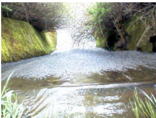
Figure 22. Site 981825 features an earthen dam with a concrete spillway at a 30% slope. This total barrier to fish passage blocks access to 2.5 km (1.57 miles) of stream containing 355 square meters of spawning habitat and 18,203 square meters of rearing habitat. The PI for this barrier is 30.61. This site is on BP land.
