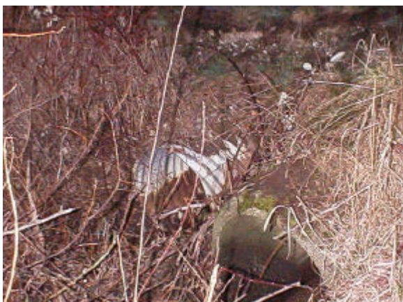
Figure 18. Site 981794. The two culverts at this site, a corrugated steel and a concrete pipe are a barrier to fish passage. This limited habitat gain site has only 179m of fish bearing stream upstream of this barrier. At 179 meters upstream, the stream flows through reed canary grass with no defined channel. The PI value is 6.85.
