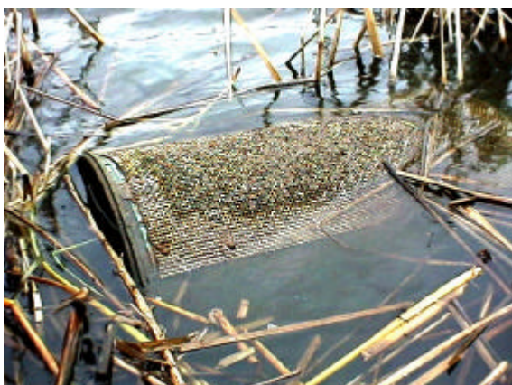
Figure 20. Site 981822 has a screened pump diversion, located in the pond created by site 981821. The screen is not compliant due to the size of the screen openings. This pump diversion supplies water during summer and fall to newly planted trees on the BP mitigation project about 250 meters to the north. No PI value could be generated because the pump was not present at the time of the evaluation.
