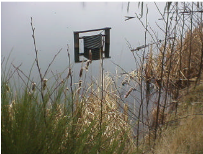
Figure 9. Site 981780, features an earthen dam with a vertical standpipe. This total barrier to fish passage blocks access to 0.26 km (0.16 miles) of stream containing 2,893 square meters of rearing habitat. The PI value for this barrier is 15.23.
