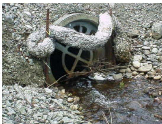
Figure 23. Site 981830, on Jackson Road, is a 0.76 m (2.50 ft) culvert. Because the upstream end is inside a high security area of the BP refinery there is a security grate installed. The worm-like mesh bag is a pollution control device. This culvert is a partial barrier due to a 2.26% slope and the PI value is 11.98. This site is owned by Whatcom County.
