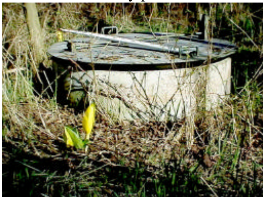
Figure 27. Site 981811. This vertical concrete culvert set in an earthen dam has slots for stop boards inside. Submerged corrugated culverts extend into and out of the vertical culvert up and downstream. There is no discernible flow going through the structure. Beaver dams divert flow around this dam making it passable during high flows. This dam partially blocks access to 14,677 square meters of rearing habitat. The PI value is 17.32.
