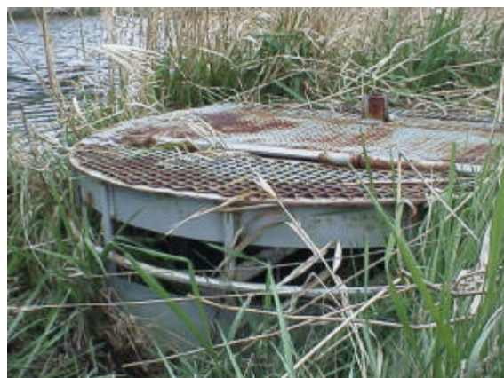
Figure 21. Site 981823 is an earth dam with a flow control structure in the dam. This pond could provide 2,392 square meters of rearing habitat. The PI value is 4.12.
