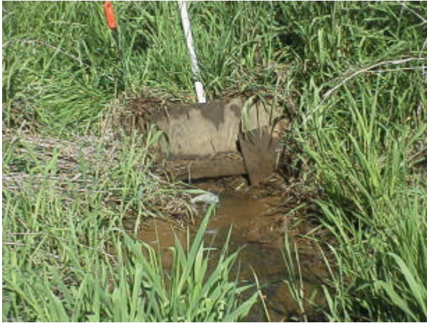
Figure 14. Site 981865 continued. View of culvert inlet, which has been boarded off.
