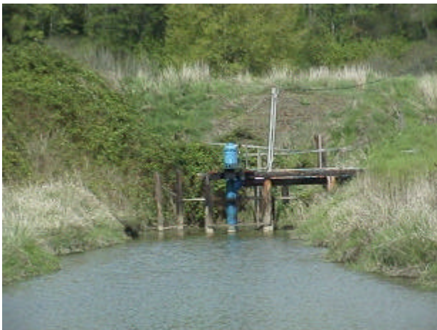
Figure 16. Site 981457, Shillapoo Lake to Lake River. View of 'expulsion' pump and sump area. The pump is unscreened and there is wire fencing being used as a trash rack.
