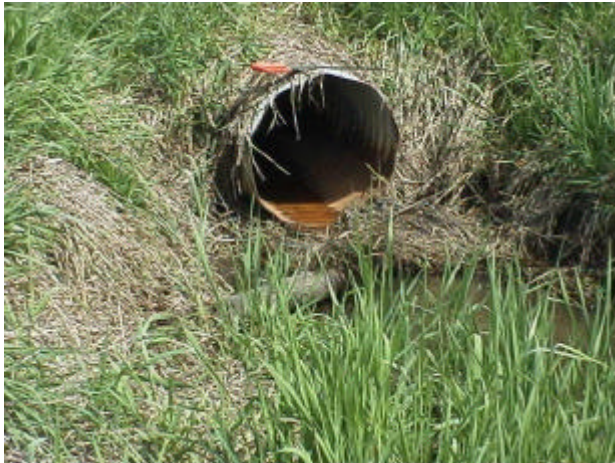
Figure 28. Site 981470, Mulligan Slough to Vancouver Lake. Set a foot higher than 981471, this site has a barrier water control structure too. This site is also a location where Mulligan Slough inundates the flood plain regularly.
