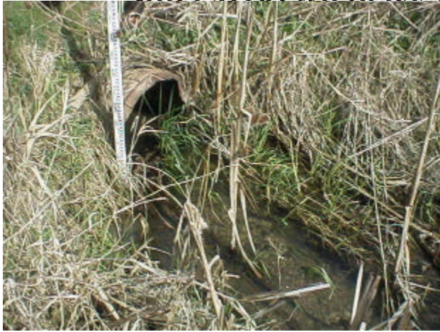
Figure 10. Site 981453, Shillapoo Lake to Lake River. This undersized culvert creates a velocity barrier. The culvert is rusted out and the upper section of the pipe is disconnected.
