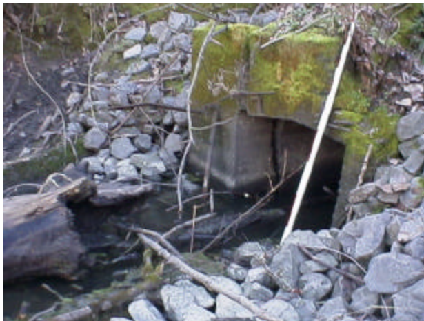
Figure 20. Site 981459, Buckmire Slough (28.0136) to Lake River. Downstream view of site. Evidence of a pre-existing tide gate was observed. The crushed rock and water control structure were recently added to this site.
