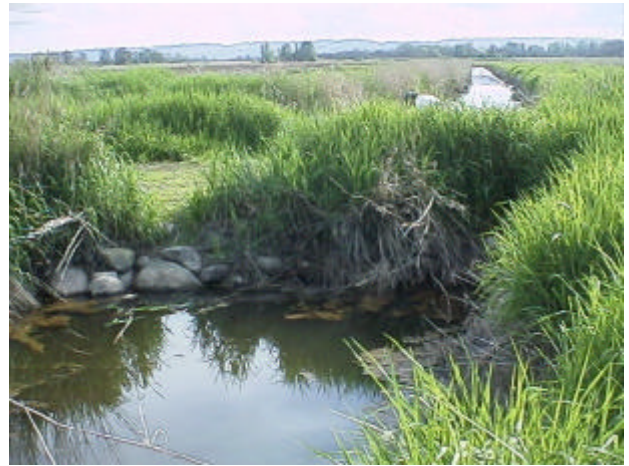
Figure 19. Site 981862, Shillapoo Lake to Lake River. This undersized culvert is a partial barrier due to velocity. The upstream end of the pipe was partially clogged when surveyed. Grazing livestock have also created water quality issues.
