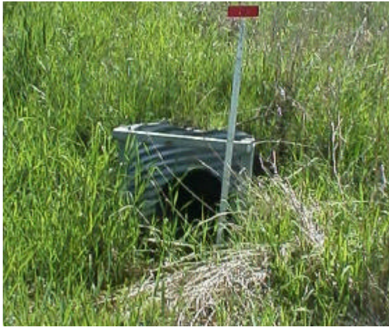
Figure 30. Site 981472, Unnamed to Mulligan Slough. View of inlet and barrier water control structure.
