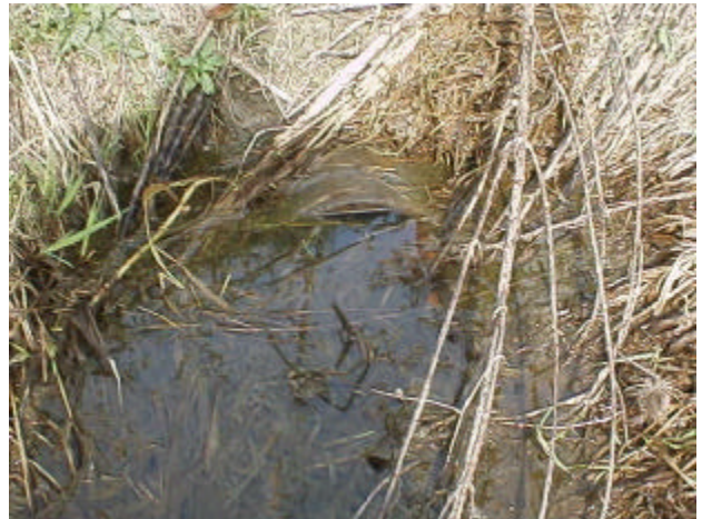
Figure 9. Site 981452 continued. Downstream view of spillway. This site is a total barrier.
