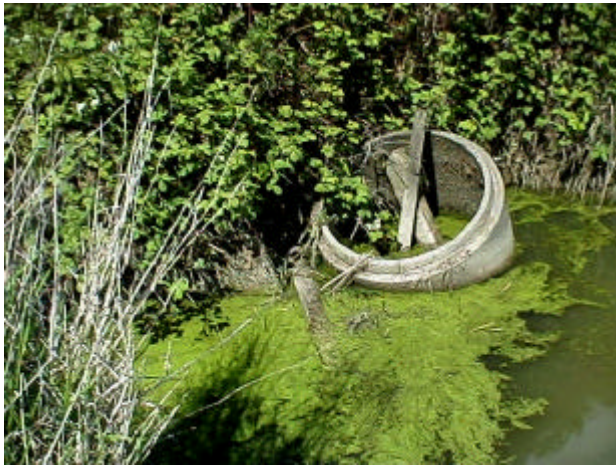
Figure 12. Site 981864, Shillapoo Lake to Lake River. Looking at the upstream end, this metal culvert is rusted out, undersized and a partial barrier due to velocity. The larger concrete round may have been dumped there.
