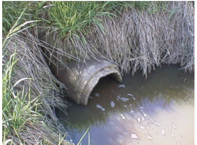
Figure 13. Site 981865, Shillapoo Lake to Lake River. This culvert has a 2.67% slope and is a total barrier.
