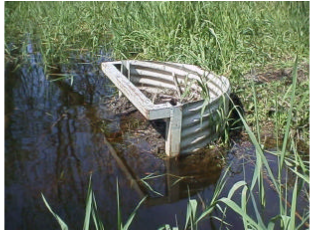
Figure 31. Site 981473, Vancouver Lake to Lake River. Beaver routinely plug this structure. The overflow levee associated with this site has a 15m wide breach that also impedes fish passage.
