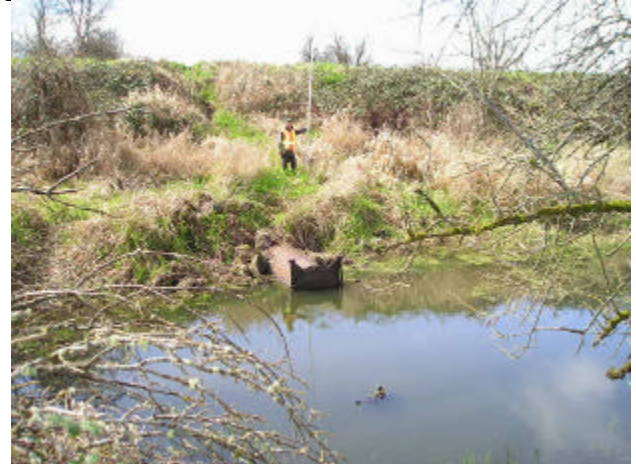
Figure 23. Site 981854, Buckmire Slough (28.0136) to Lake River. This site is a barrier culvert due to the tide gate. The hinges on the tide gate are rusted, but appear operable.
