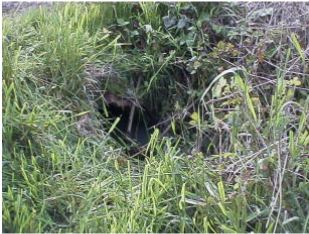
Figure 18. Site 981861, Shillapoo Lake to Lake River. Located on a ditch that is fed by a natural spring, this undersized culvert is a partial barrier due to velocity.
