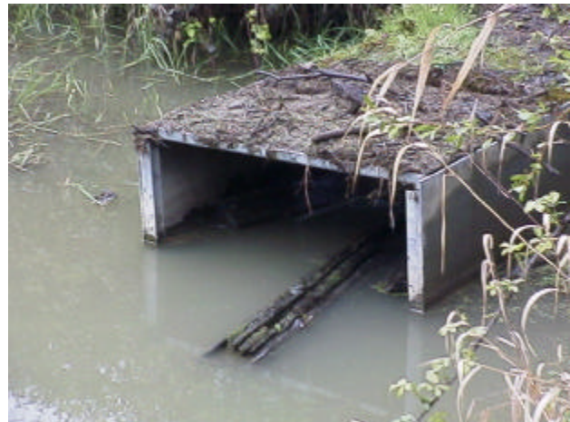
Figure 21. Site 981459 continued. View of water control structure upstream. With no dam boards installed and a water depth of 0.51 meter, the culvert is passable under these conditions. When water is held back, a barrier outfall drop is created.
