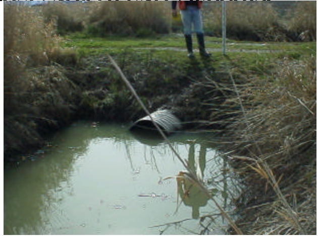
Figure 11. Site 981454, Shillapoo Lake to Lake River. Located in a drain canal, this culvert has a 2.39% slope and is a partial barrier.
