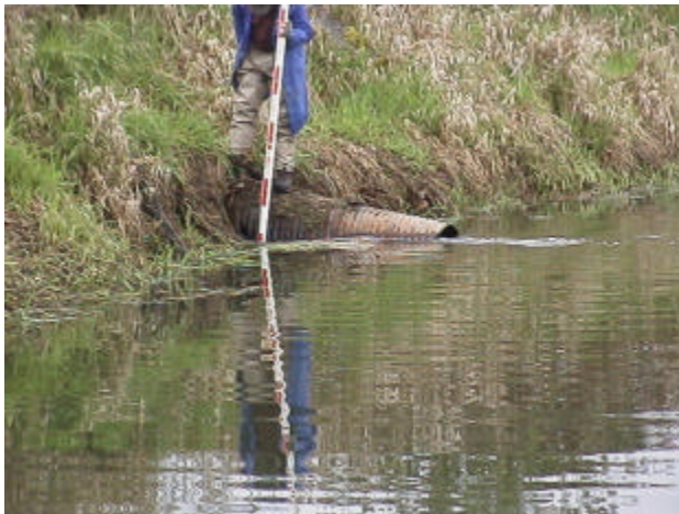
Figure 24. Site 981855, Buckmire Slough (28.0136) to Lake River. Downstream view of the mid-channel culvert at this crossing. With a slope of 1.16% and receiving the majority of the flow, this undersized culvert is a partial barrier. The sides and bottom of the culvert are rusted out. Both ends of pipe are collapsed as well.
