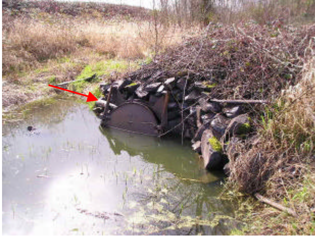
Figure 22. Site 981853, Buckmire Slough (28.0136) to Lake River. Under State Route 501, this crossing is a barrier culvert due to the tide gate. The flap style tide gate is currently propped open with LWD.
