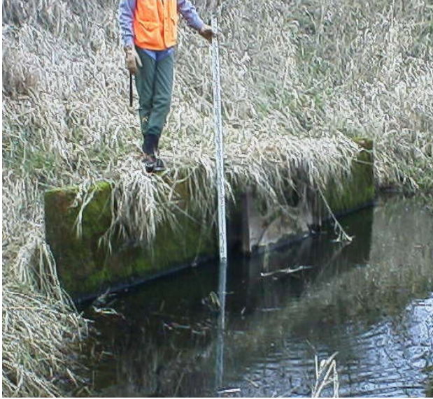
Figure 6. Site 981451, Shillapoo Lake to Lake River. This barrier culvert is fitted with a tide gate and has a 2.64% slope. Photo shows inundation from Lake River at high tide.
