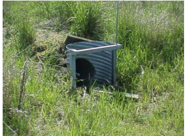
Figure 29. Site 981469, Unnamed to Mulligan Slough. View of inlet and barrier water control structure.
