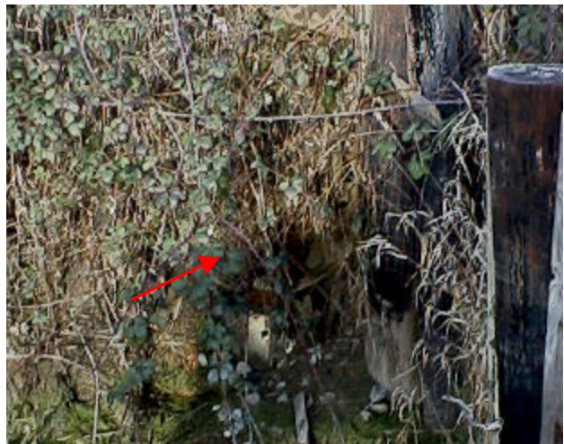
Figure 17. Site 981457 continued. Upstream view of tide-gated discharge pipe. Flow and fish access through this pipe is unknown. This location is a human made outlet for Shillapoo Lake.
