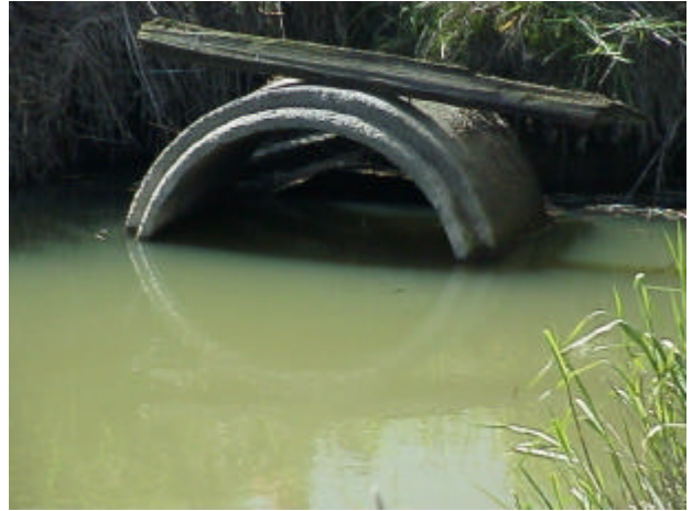
Figure 15. Site 981866, Shillapoo Lake to Lake River. This undersized (0.80 meter round metal) culvert has a larger concrete round placed at the outlet and is a partial barrier due to velocity. Scoured fill was observed at the upstream side and on top of the crossing.
