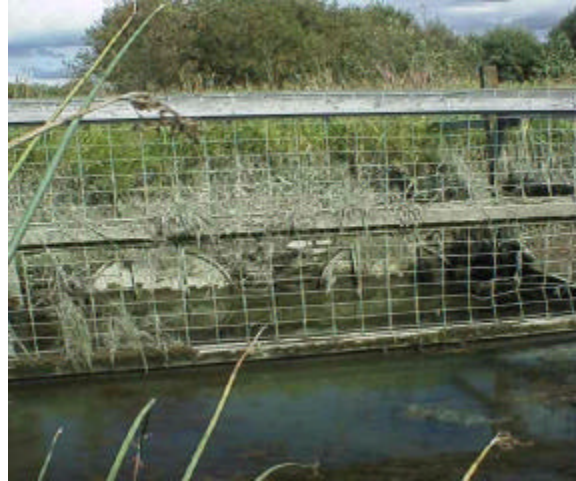
Figure 7. Site FI 15 continued. Left bank picture shows 2 of 6 culverts with tide gates. This site is a partial barrier.
