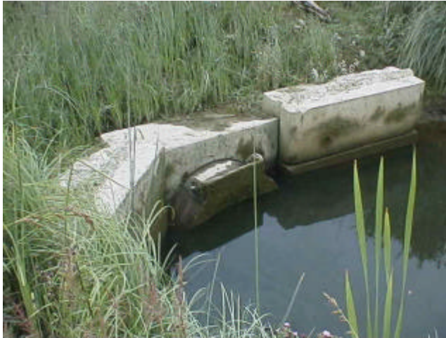
Figure 10. Site FI 9. Dry Slough to Skagit Bay. View of right bank tide gate. This site is a partial barrier.
