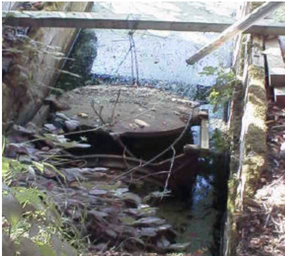
Figure 8. Site FI 19. Teal Slough to Wylie Slough. Downstream view of wired open tide gate. Upstream screw gate for wetland enhancement not shown. Currently, several metal fence posts are positioned in the channel at the inlet to prevent beavers from clogging the structure.
