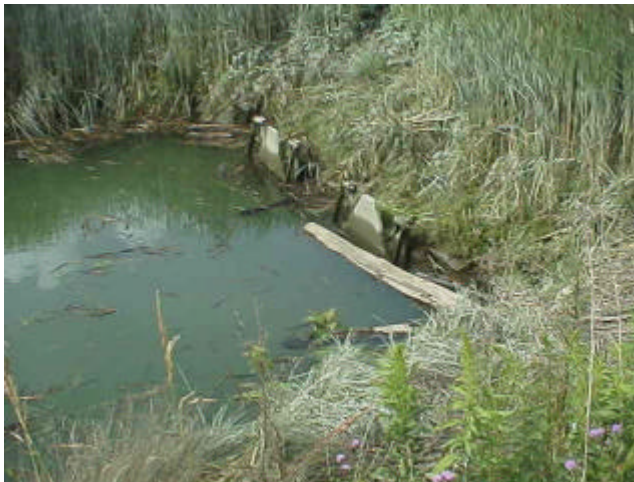
Figure 12. Site FI 41, Unnamed slough to Skagit Bay. View of partial barrier flap-style tide gates.
