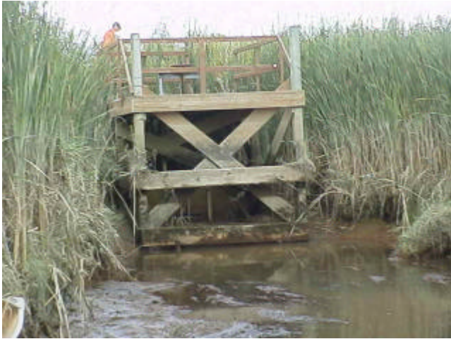
Figure 14. Site 981874. View of combination drainage and canal gate with platform to access the handwheel for raising the gate to allow backflow. Fish passage is dependent on management activities.
