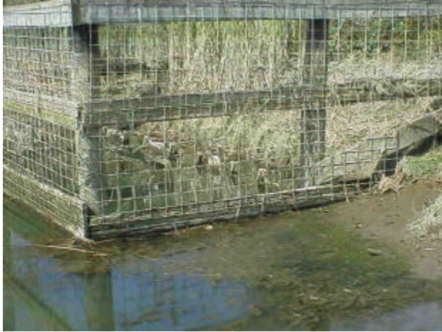
Figure 6. Site FI 15. Wylie Slough to Skagit Bay. Right bank picture shows 4 of 6 culverts with tide gates. All 6 gates are of the flap style.
