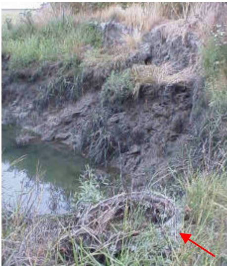
Figure 16. Site 981916, Unnamed to Davis Slough. Downstream view of eroding dike and remnant tide gate in the bank.
