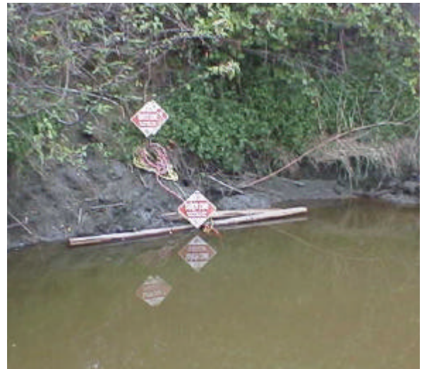
Figure 17. Site 981916 continued. Upstream view shows the orange tube for the air bladder apparatus used to plug the culvert until repairs can be made.
