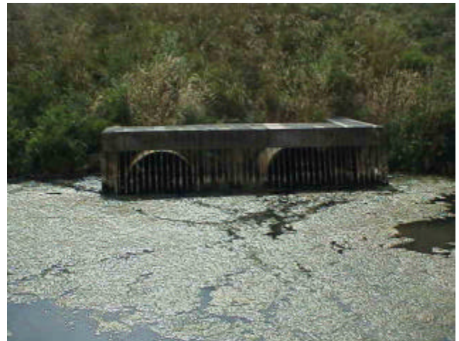
Figure 13. Site FI 41 continued. Upstream view shows trash rack structure and stagnant water.
