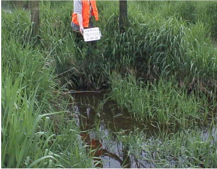
Photo 6. Unnamed tributary to Cherry Creek. Located on a dead end drainage ditch, this barrier culvert is completely inundated with silt and vegetation. Repair would allow fish passage to and from additional winter rearing habitat.
