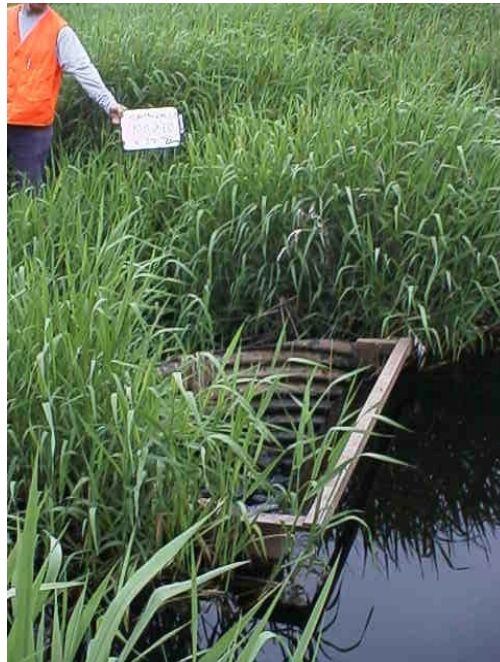
Photos 4. Unnamed tributary to Cherry Creek within the drainage ditch system. The upstream end of the culvert is fabricated with a pond level control structure to increase waterfowl habitat. Currently, it is a partial barrier to fish migration and requires repair in order for migrating fish to reach available spawning habitat.
