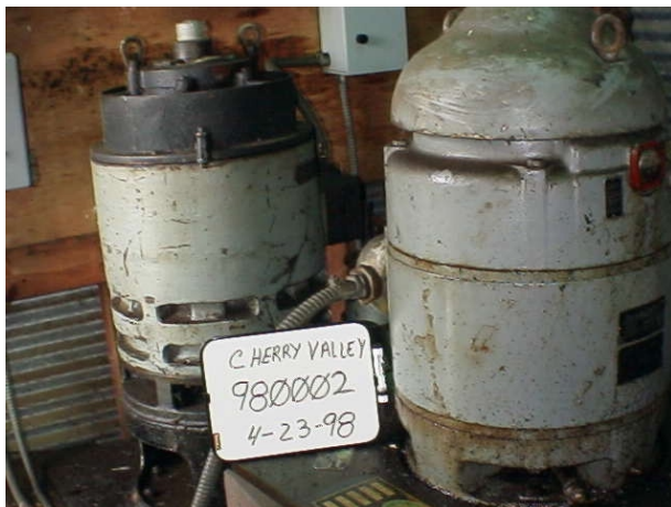
Photo 3. Pump motors inside pump house.
