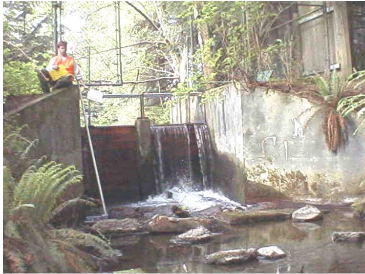
Photo 21. Tulalip Creek (07.0001). The feature was originally designed as a drum screen lake outlet structure. The screen has been removed and the structure is currently used as a lake level control device. It is a total barrier and requires repair.
