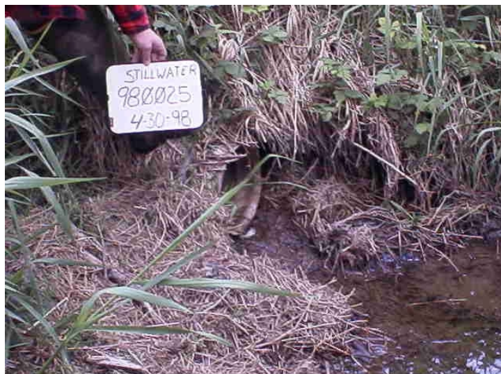
Photo 11. Unnamed tributary to Snoqualmie River. Located on the same tributary as site 980024, this small corrugated steel culvert is undersized and influenced by heavy beaver activity. If repaired additional winter rearing habitat would be accessible.
