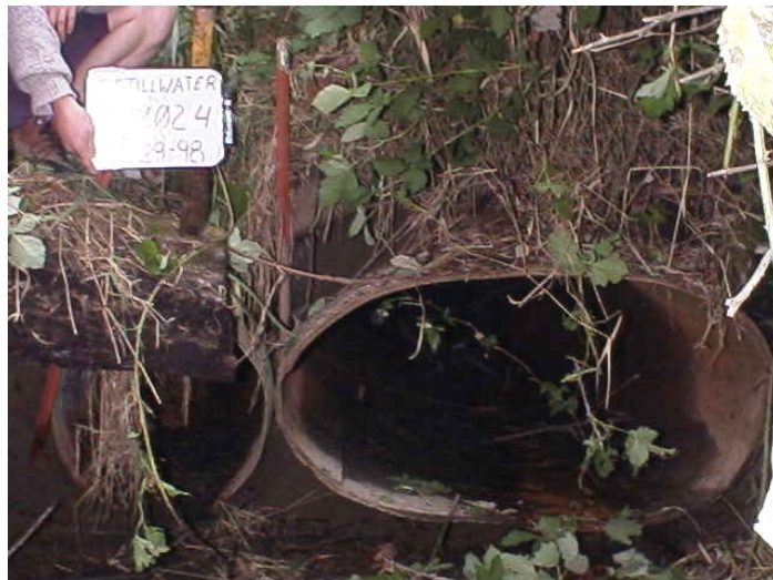
Photo 10. Unnamed tributary to Snoqualmie River. Even though two culverts have been used at this crossing, during winter flow, it is still undersized. Repair would allow access to additional winter rearing habitat.
