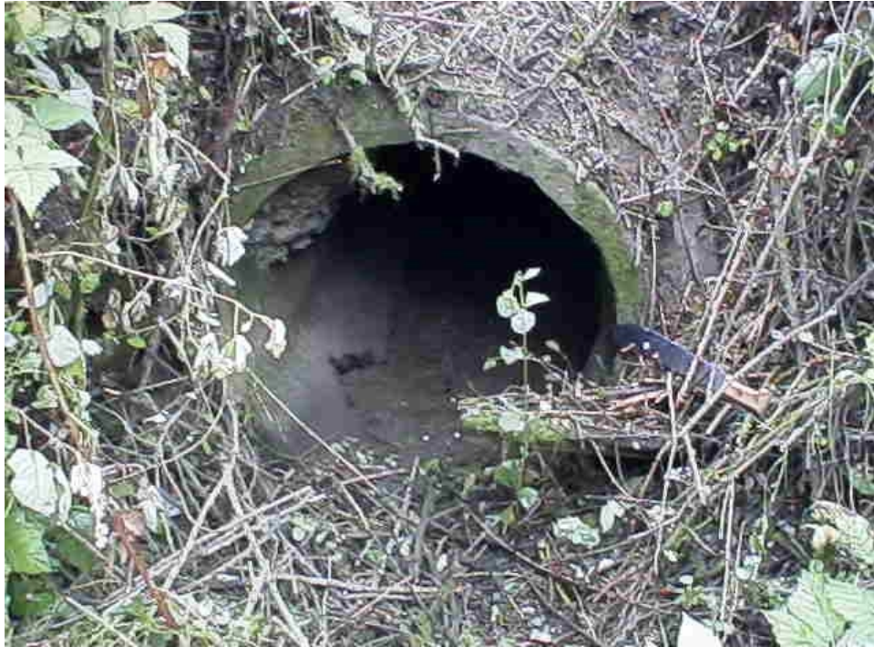
Photo 13. Unnamed tributary to Snoqualmie River. This round concrete culvert is located on the same tributary as Site 980027 and is severely undersized for winter flows. A huge plunge pool has formed due to the velocities the culvert creates. Again, the primary benefit in replacing this culvert is for winter rearing habitat.
