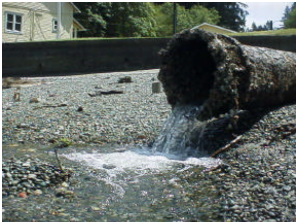
Figure 11. Site 981751. Luhr Creek barrier culvert outlets directly into Puget Sound. This 40 meter long, 0.31 meter diameter culvert is a total barrier to fish passage.
