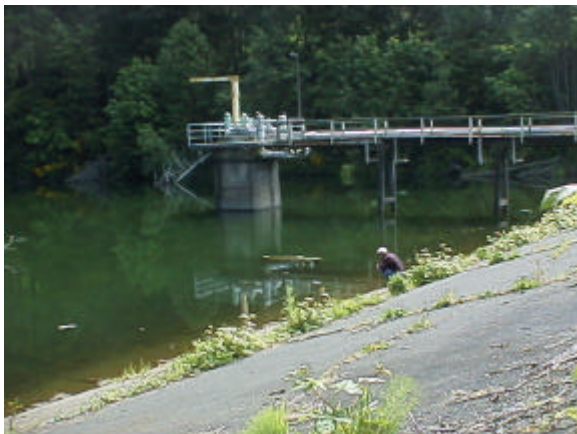
Figure 7. Site 981735. Eden Creek Dam, Reservoir and pump equipment. Water is pumped to a water treatment plant.
