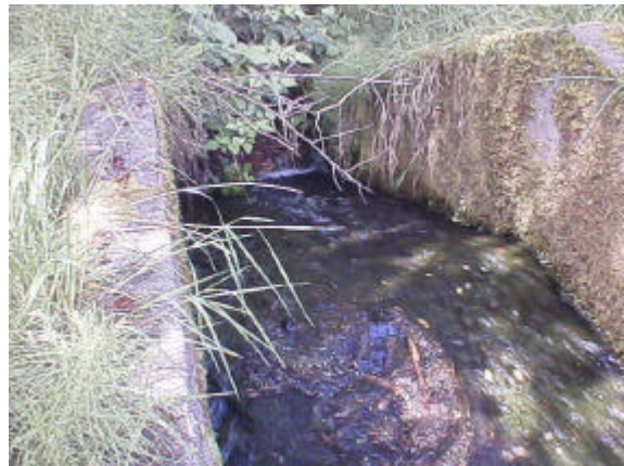
Figure 12. Site 981750. About 60 meters upstream of site 981751 is Luhr Creek dam and spillway. The spillway, pictured above, is a total barrier due to slope and sheetflow.
