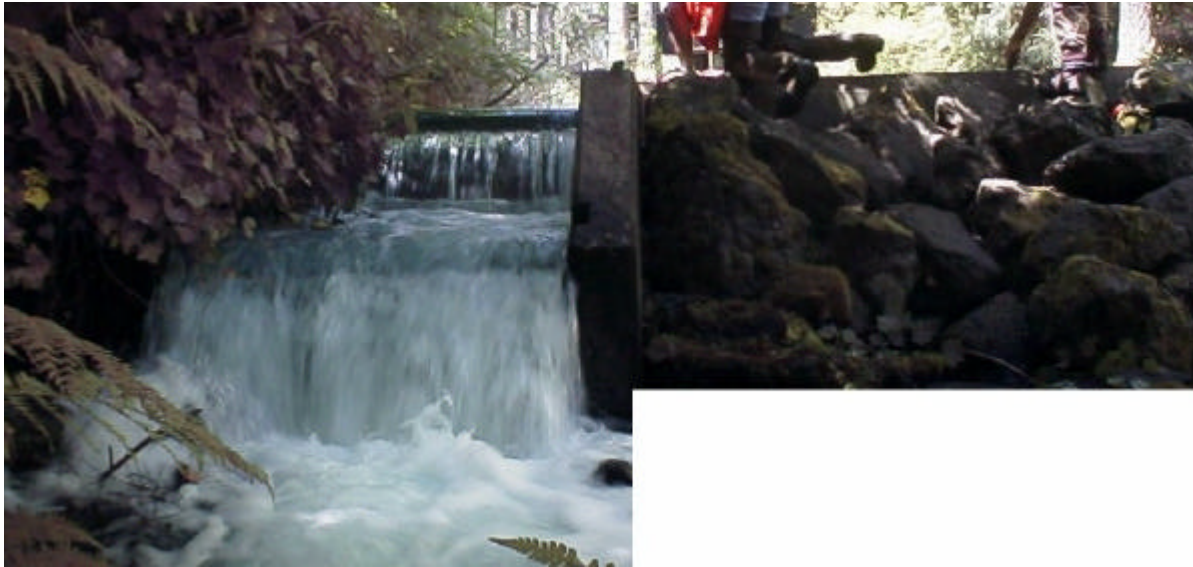
Figure 6. Site 981870. This concrete dam and fishway partially block access to 237 meters of stream habitat. The outfall drops on the fishway are 0.50 meters and 0.51 meters. Trout were observed in the upstream pool. This stream is the outflow from the Lakewood Fish Hatchery.
