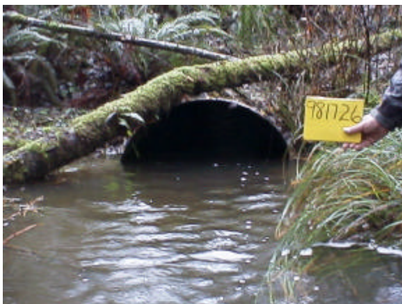
Figure 17. Site 981726. Unnamed tributary to Scatter Creek. This 1.12 meter diameter culvert is a barrier due to a 1.35 percent slope.
