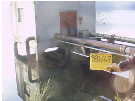
Figure 10. Site 981767. Offshore intake pumps Butterworth Reservoir water to the North Facility Complex.
