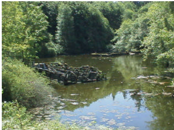
Figure 16. Site 981770. Milewa Creek Reservoir is about 1.0m above the high tide line of Puget Sound. An overflow culvert spills water into the Sound.
