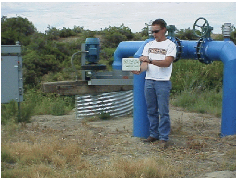
Photo 4. Example of a “lift” pump diversion configuration. Recently installed on the Sunnyside Unit for controlling water levels of Bos Lake and/or Horseshoe Pond, this pump system has an unscreened intake submerged in DID #7.
