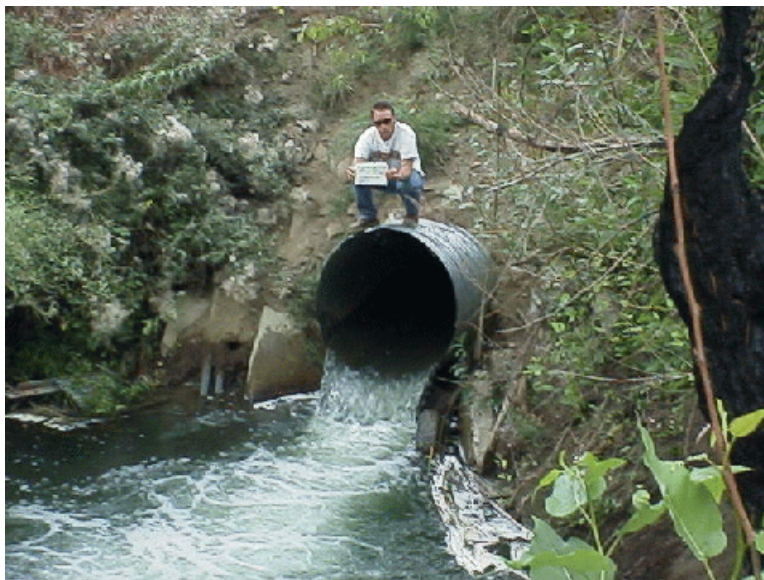
Photo 1. Lowest barrier culvert on the DID #7 drainage. Although the culvert slope is less than 1%, this culvert is a barrier due to excessive outfall drop and high velocity. It is also undersized.
