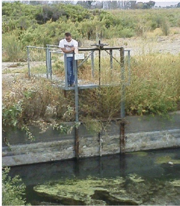
Photo 2. Upstream end of the diversion dam. Site is a partial barrier due to control structure. With the screw gate partially open and the current flow conditions, the culvert (spillway) was determined to be passable at time of evaluation.
