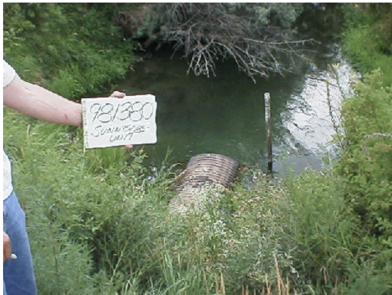
Photo 3. The downstream end of culvert at Site 981380 better illustrates size of culvert in comparison to channel width. Notice the makeshift flow gauge used to monitor and manipulate water levels.
