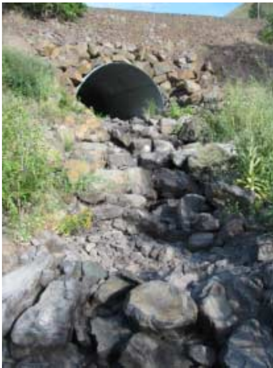
Photo 1. Lower culvert with a steep delta and rock weirs in lower Grouse Creek that is 100 meters or more upstream of the Grande Ronde River during summer.
