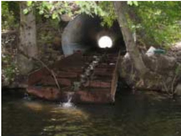
Photo 9. Culvert (6-8 ft in diameter) and fish passage apron just downstream of the Oregon state line on Washington Highway 129 (becomes Oregon Highway 3) on Buford Creek. Large deep pool below culvert upstream of site BU-1.
