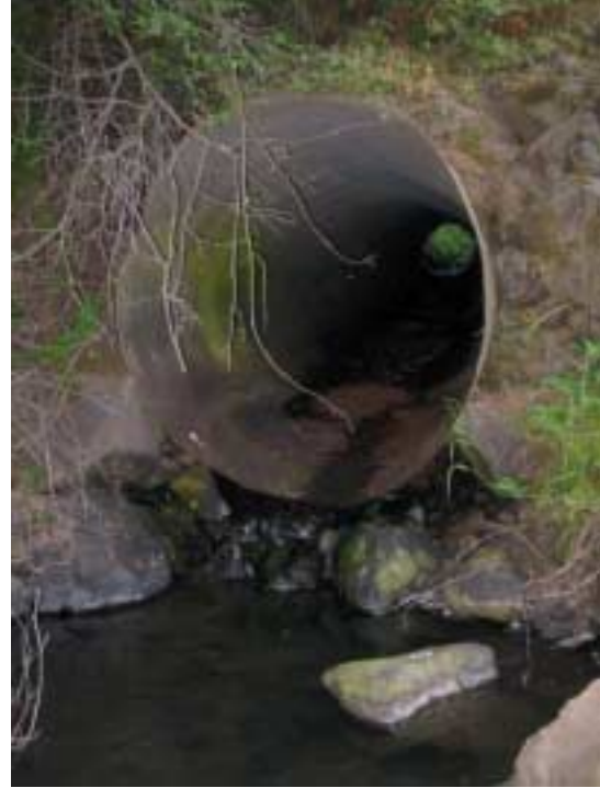
Photo 4. Long, steep culvert (Second culvert upstream of mouth of Grouse Creek) that is rusted through 0.5 meters from the downstream end. Much of the water during low flow goes under the lower portion of the culvert instead of discharging at the bottom lip of the culvert. This culvert is in need of replacement.
