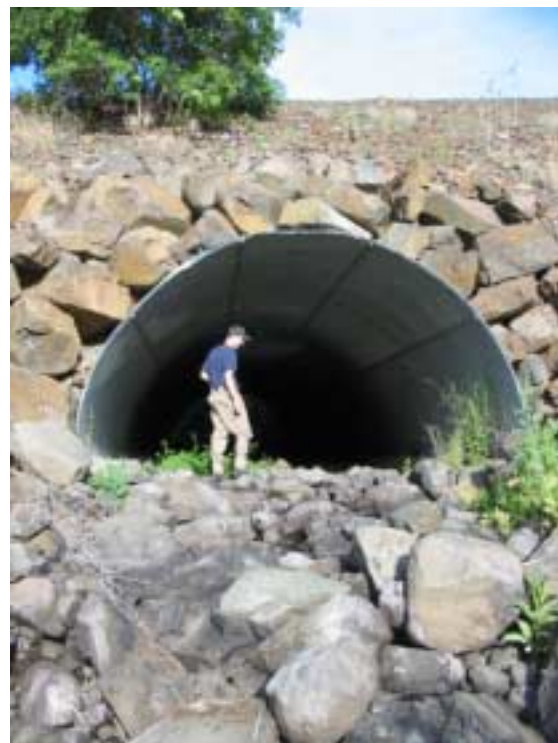
Photo 2. Lower Culvert (in Photo 1) and its relative size at roadway to Troy, Oregon.
