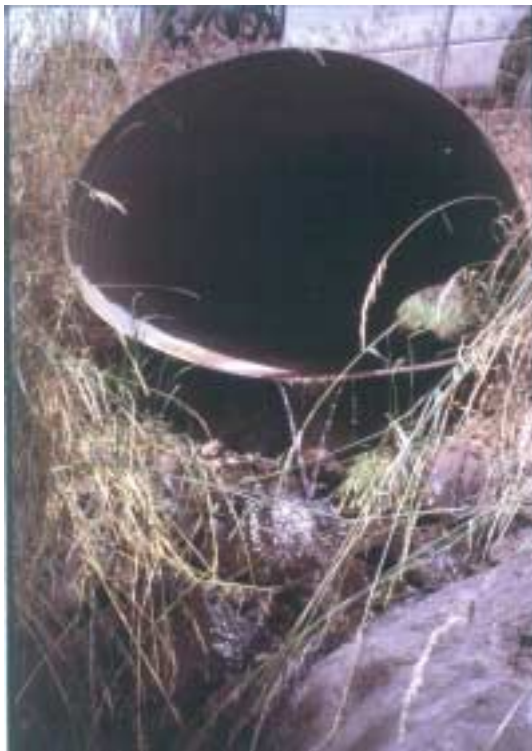
Photo 16. Culvert on upper Shumaker Creek at low flows. It appears to be a total barrier, even if flows were higher.
