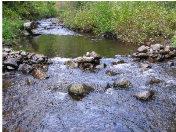
Photo 176. Man-made rock dam in the North Fork Wenaha River after surveyors notched it for fish passage, September 2007.
