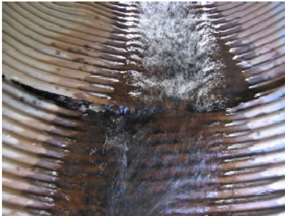
Photo 32. Shumaker Creek at first culvert above mouth looking at gap in two sections of culvert (SH-2), April 2007.
