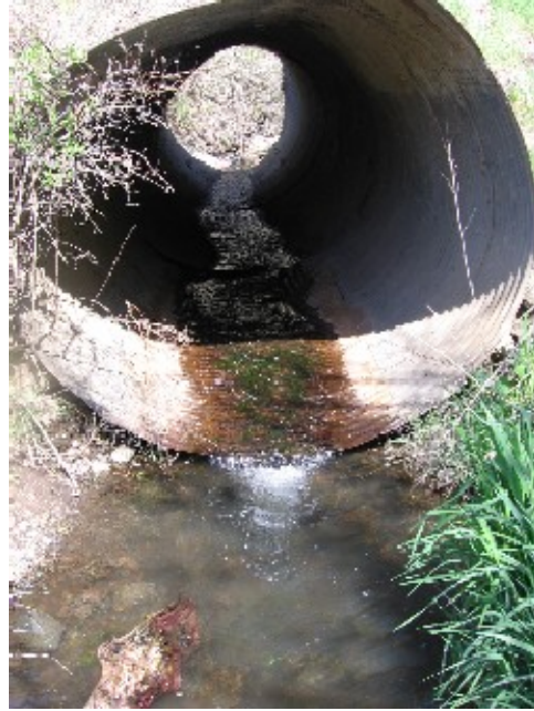
Photo 31. Shumaker Creek at first culvert above mouth looking up into culvert (SH-2), April 2007.
