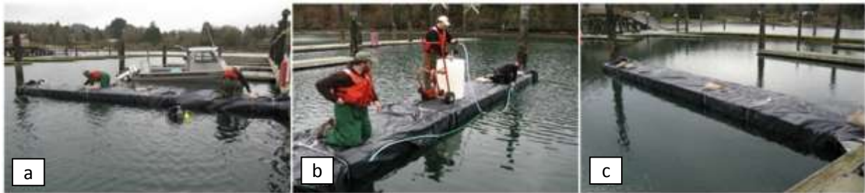
Figure 5. a) SCUBA divers and surface personnel encapsulating a dock with polyethylene plastic. b) Pumping 20% acetic acid into the encapsulation. c) Completed wrap with acetic acid infusion.
