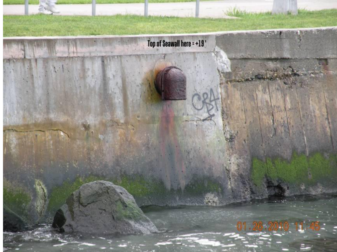
Run-off outflow pipe noted near Station three of EBDH. Photo taken prior to low tide sampling window.
