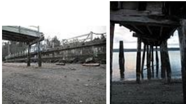
Creosote pilings of old ferry terminal and cement retaining near PSHC site.
