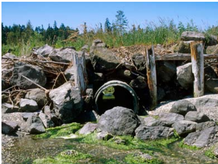
Pitship Before: Undersized culvert that was blocking tidal and fish access at Pitship Pocket Estuary in Sequim Bay
