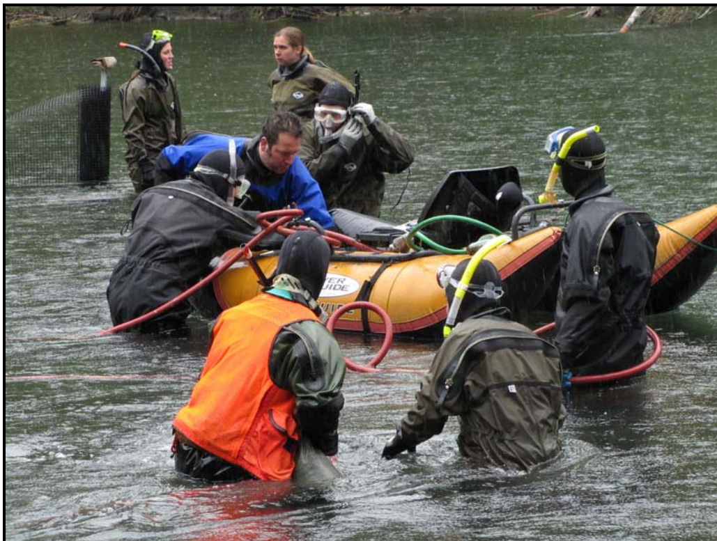
Equipment used in-river during installation of the floating weir in the Elwha River (2010).
