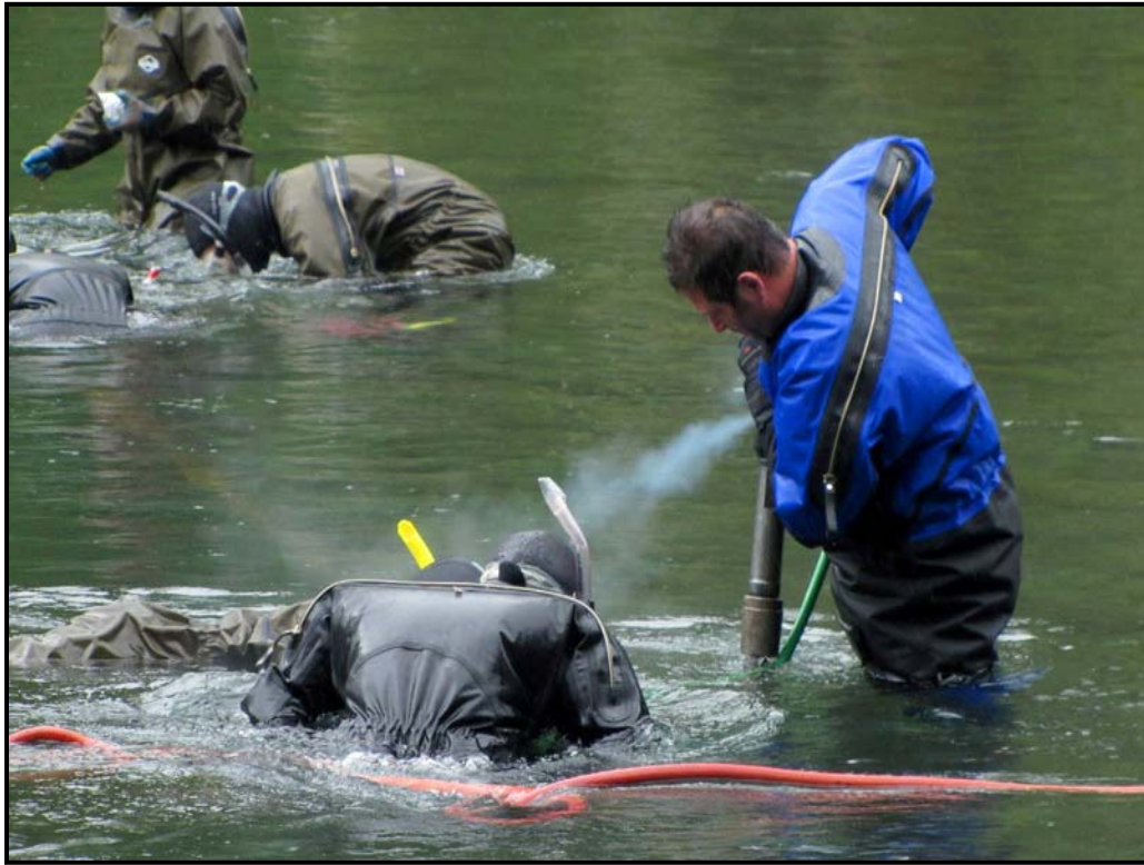
Driving pins during installation of the floating weir in the Elwha River (2010).
