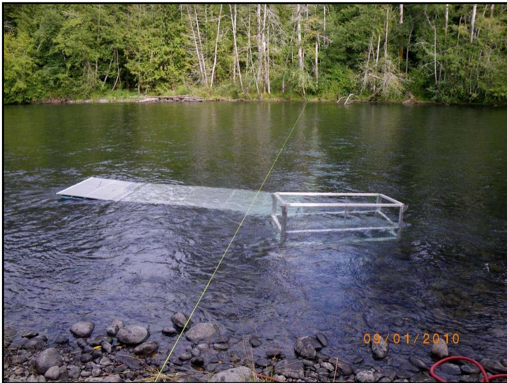
First two panels used during installation of the floating weir in the Elwha River (2010).
