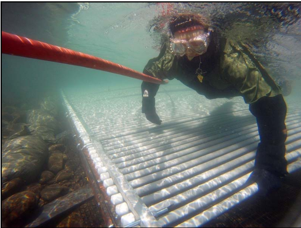
Adjusting panels during installation of the floating weir in the Elwha River (2010).
