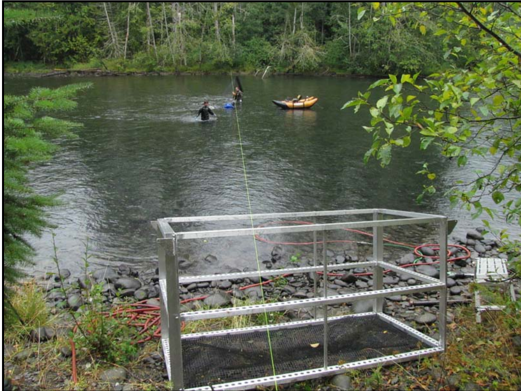
Rail set line used during installation of the floating weir in the Elwha River (2010).
