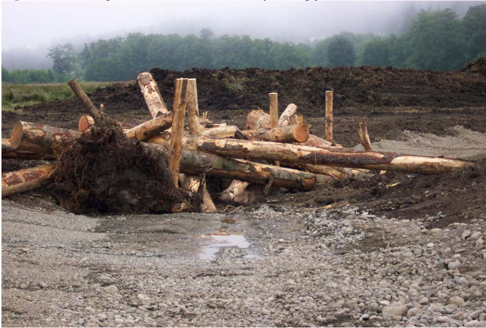
Figure 11. Piling used to increase stability of log jam (Salmon Cr, Jefferson Co., WA).
