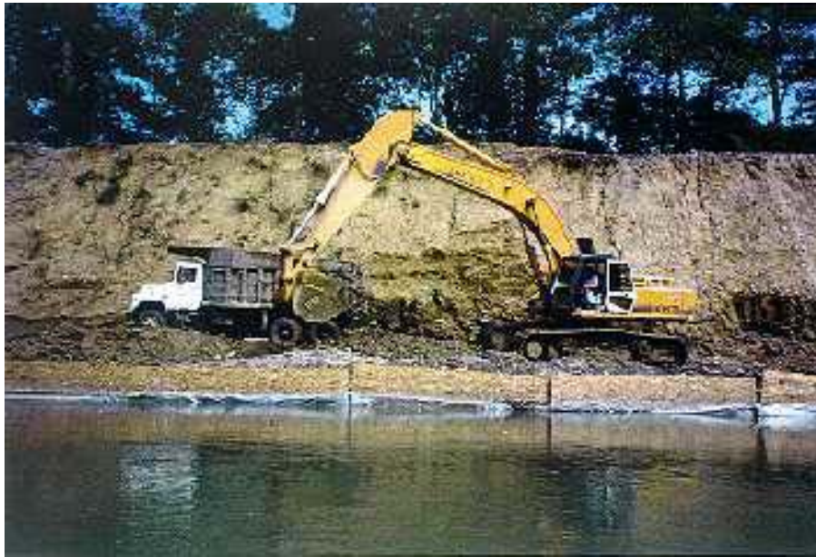
Figure 3. Construction platform for major streambank restoration, Little Miami River, Ohio. Source: Inter-Fluve, Inc.
