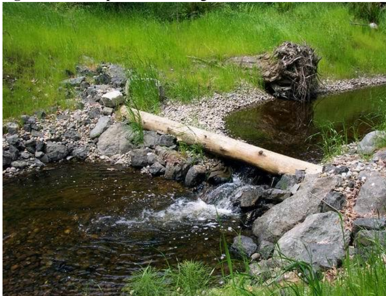
Figure 9. Example of failed log/rock weir.
