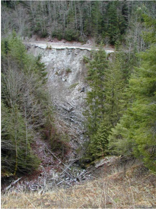
Figure 3. Erosion initiated by poor road drainage. Source: Paul Bakke
