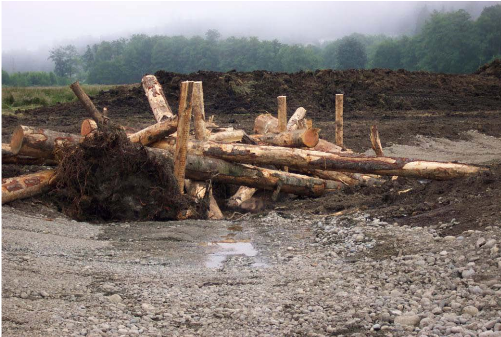
Figure 13. Logs with tapered tips installed with impact pile driver (Cowlitz River, WA, Inter-Fluve, Inc.).
