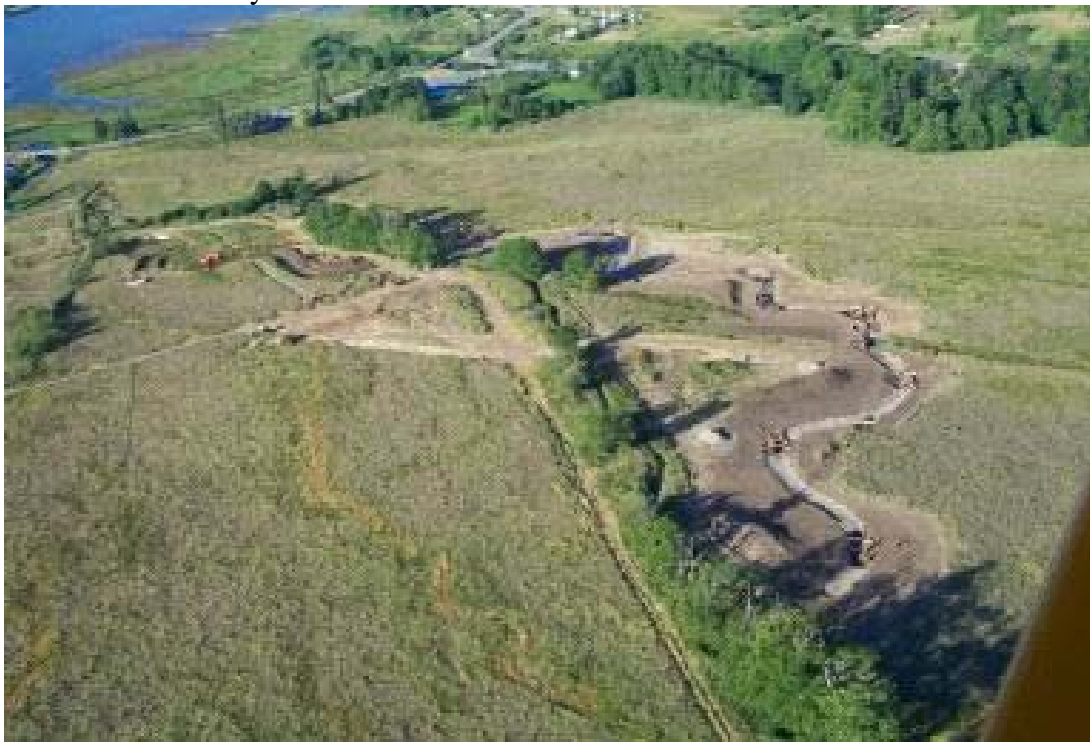
Figure 5. Aerial view of Salmon Creek project under construction. Photo provided courtesy of the Jefferson County Conservation District.
