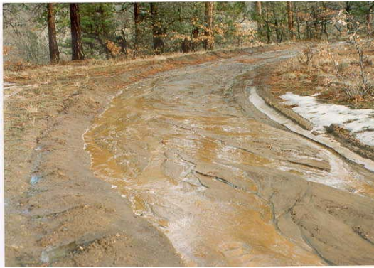
(a) Surface erosion from a road
