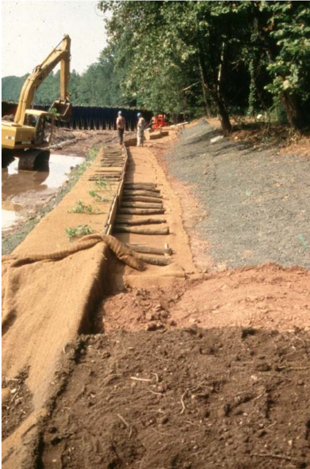
Figure 7. Installing rooted willow cuttings during fabric encased soil lift construction. Source: Inter-Fluve, Inc.
