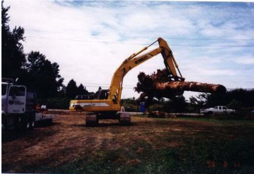
Figure 8. A track hoe excavator manipulating a large root wad and bole. Source: Inter-Fluve, Inc.
