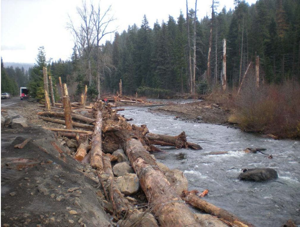
Figure 9. Bank protection using large wood anchored by a combination of techniques; rock ballast, cabling, and pilings (Klickitat River, WA, Inter-Fluve, Inc.).
