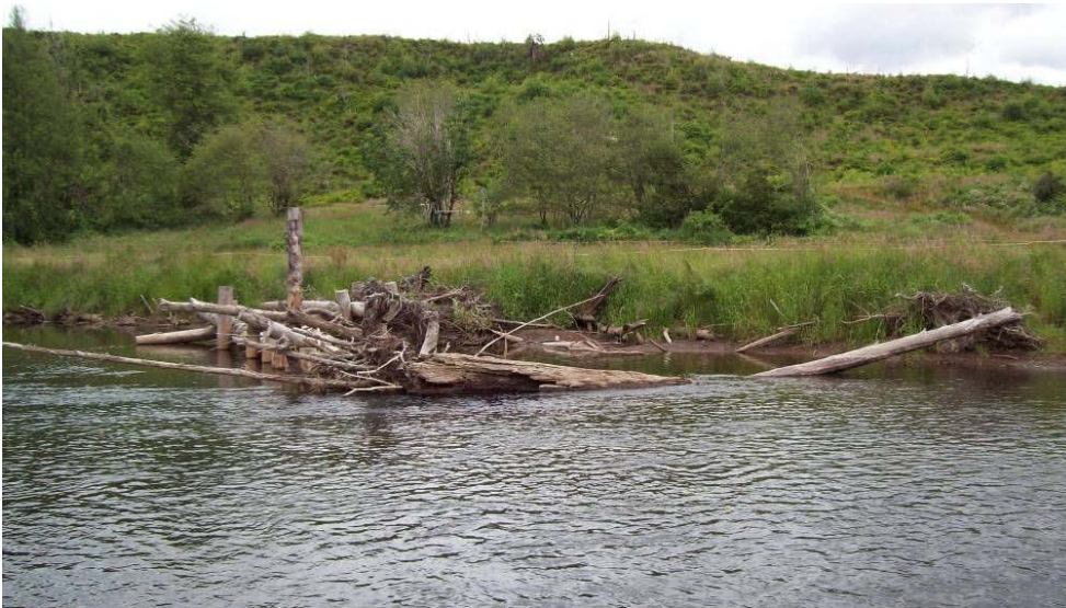
Figure 12. Log pinned to installed piles (Grays River, WA, Lower Columbia Fish Enhancement Group).
