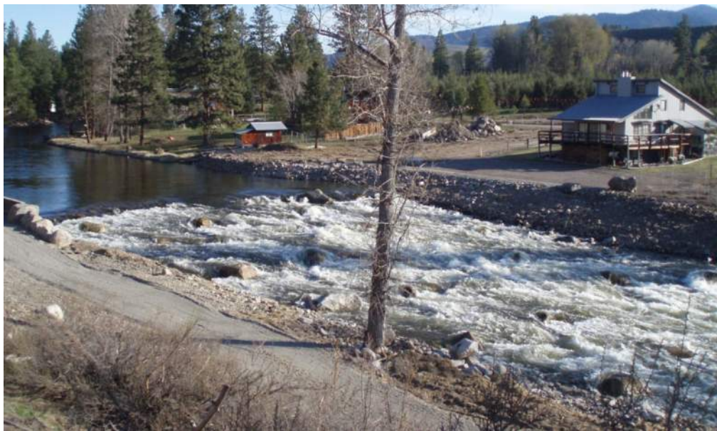
Figure 6.5: Fulton irrigation diversion with roughened channel. Irrigation intake is to the left in the photo. This type of roughened channel is often referred to as a rock ramp and its design has been described by Aadland (Bates and Aadland 2006) and Newberry (Newbury and Gadoury 1994).
