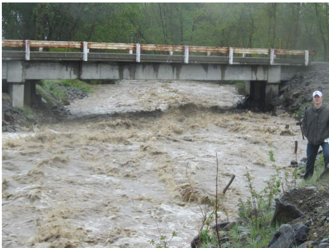
Figure 6.7: Taenum Ck. Bruton irrigation diversion. This roughened channel is shown at high flow. The design must consider flow conditions like this to ensure that the channel does not degrade. Photo Paul Tappel.
