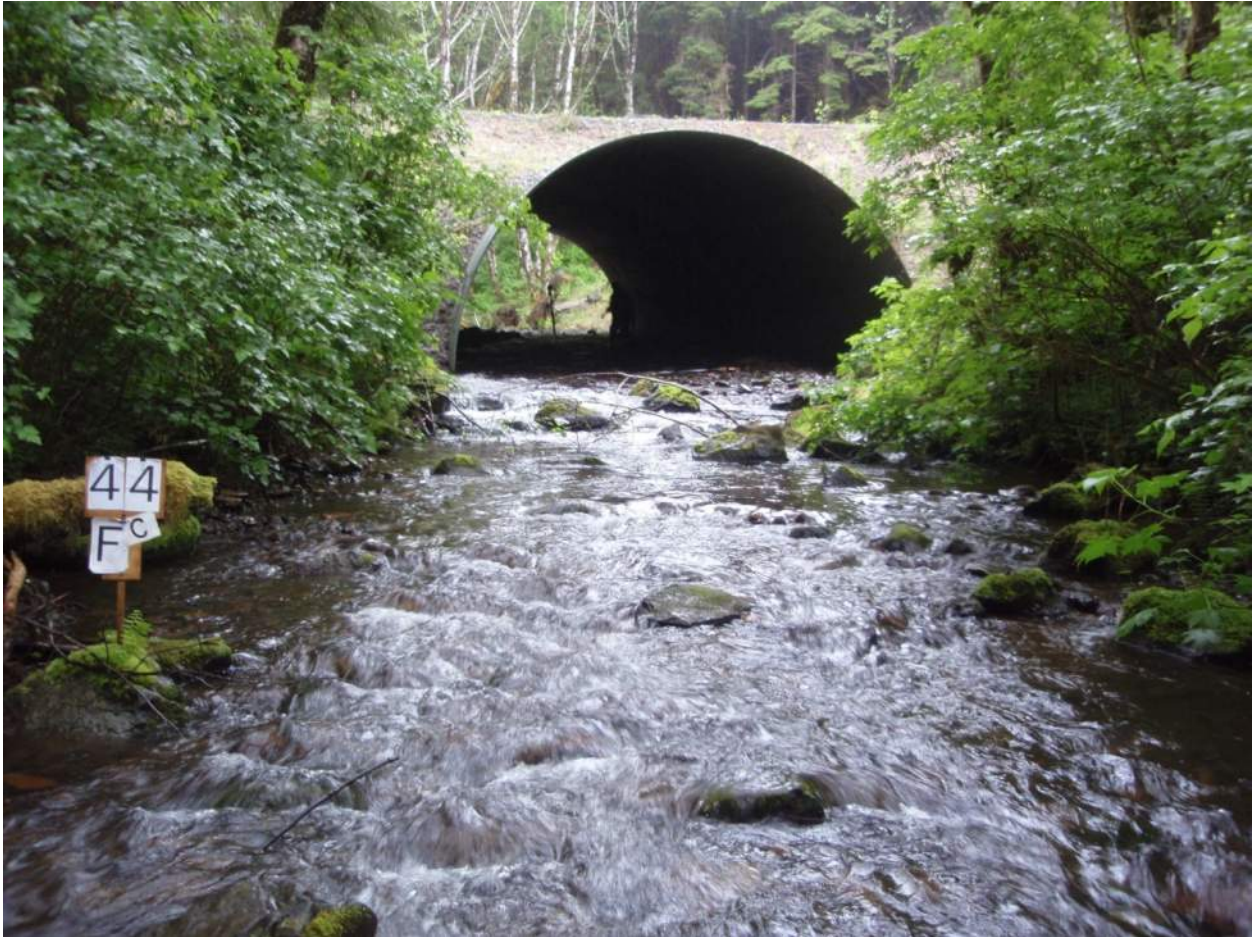
Figure 3.1: Stream simulation culvert, Newberry Ck.
