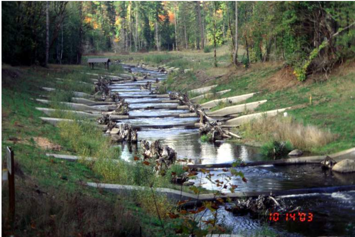
Figure 7.6: Soldier pile and cast concrete grade control structures at a dam removal site on Goldsborough Ck. This site has now become thickly vegetated and has a more stream-like appearance.
