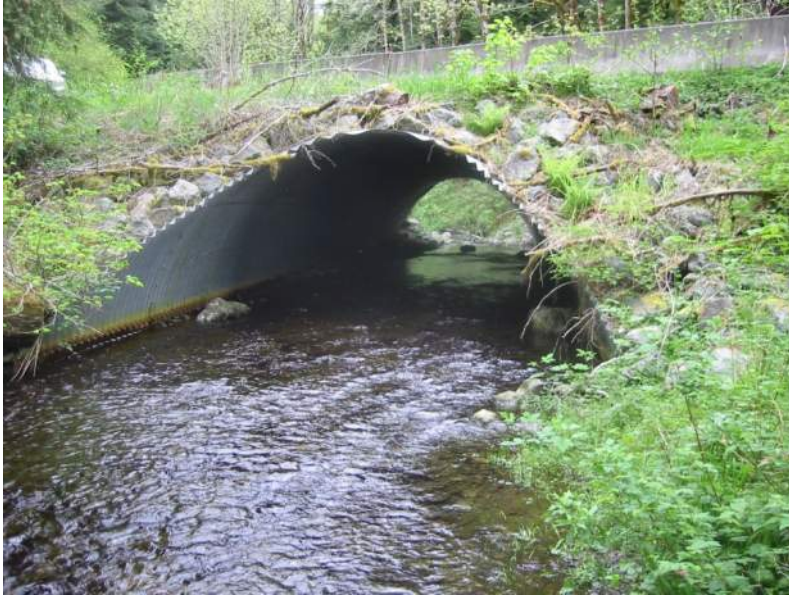
Figure 2.1: No-slope culvert, Johnson Ck, Mosquito Lake Rd.
