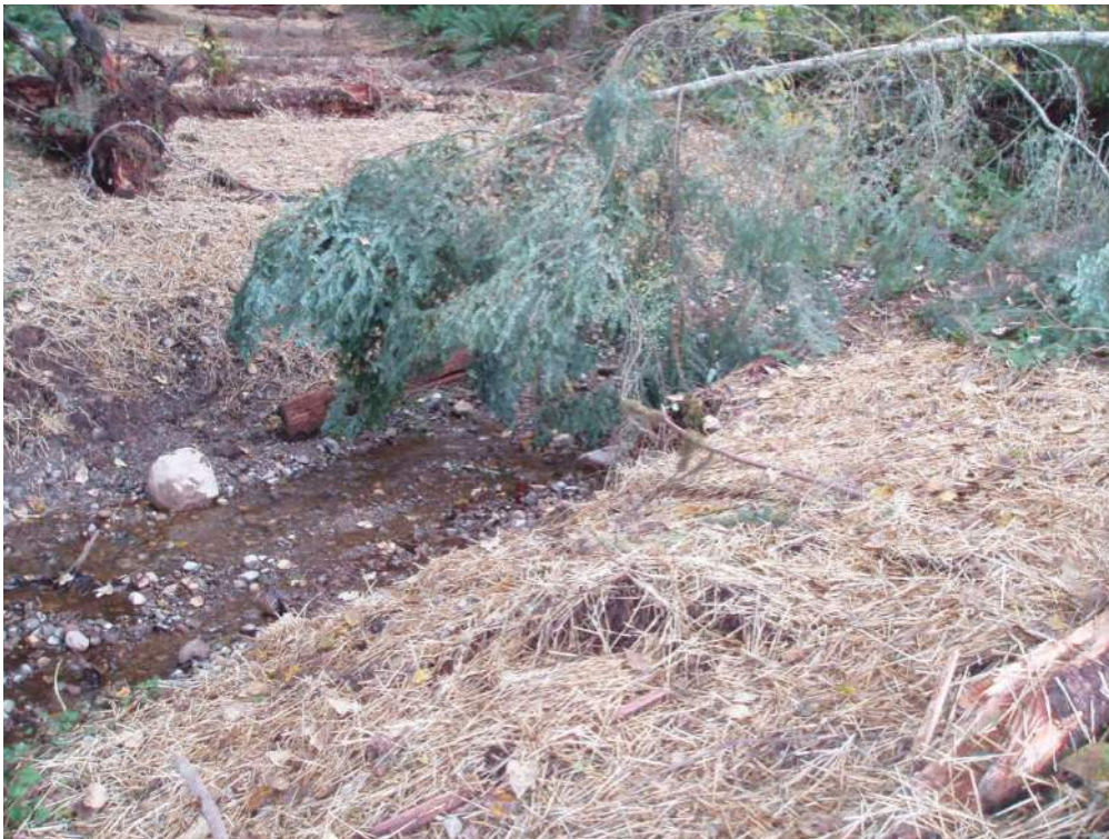
Figure 8.2: Temporary culvert site after removal. All traces of the temporary fill are removed and straw is placed on the banks to decrease erosion. Wood and slash are added to improve habitat.
