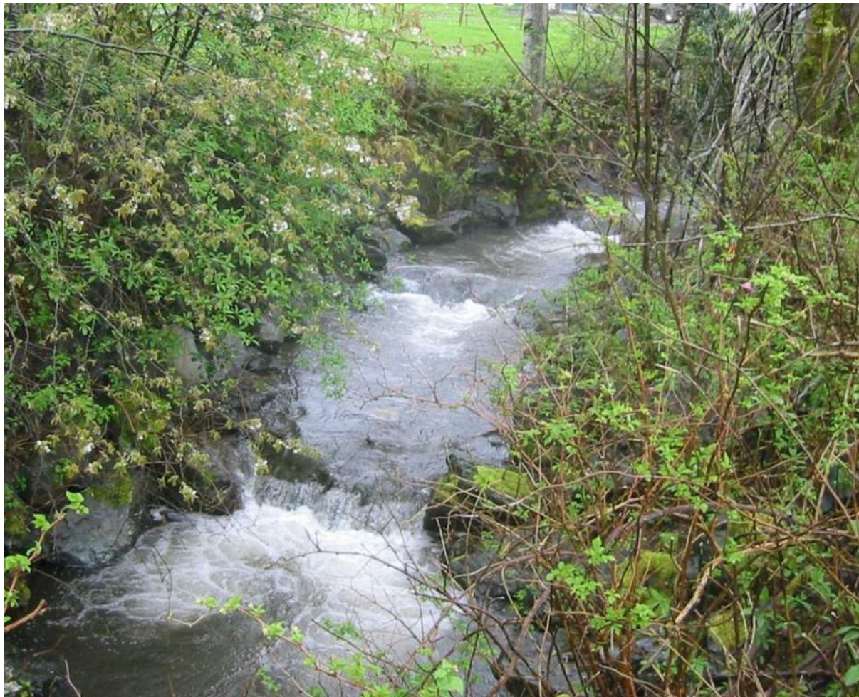
Figure 7.8: Boulder controls to maintain grade at a culvert replacement site, NP Ck. These controls are 13 years old.
