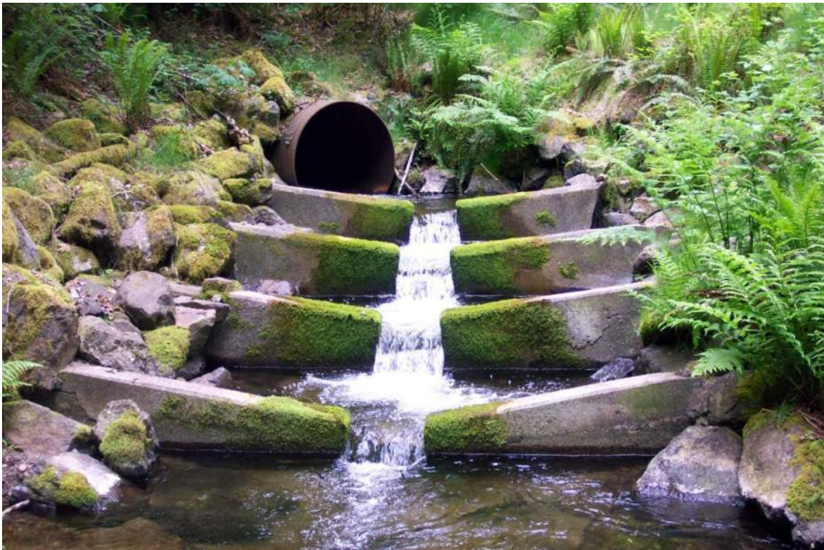
Figure 7.9 Fishway at the outlet of a baffled culvert, Dickerson Ck. This fishway is composed of precast concrete weirs formed to a pool and chute configuration.
