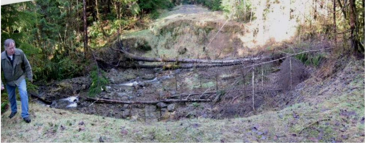
Figure 8.1: Culvert abandonment site showing full floodplain excavation and placement of large wood in excavation.
