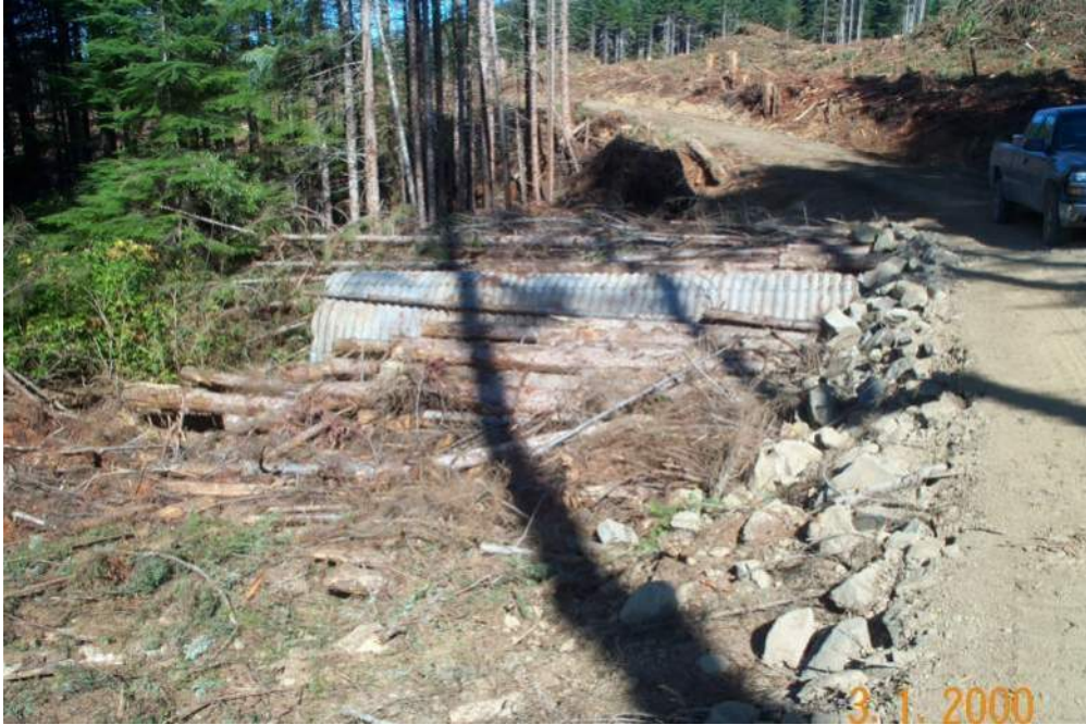
Figure 8.1: Temporary culvert. Non-merchantable logs are used as fill around the culvert to make it easier to remove and to protect the culvert. Road fill is kept to a minimum and native soils are used.
