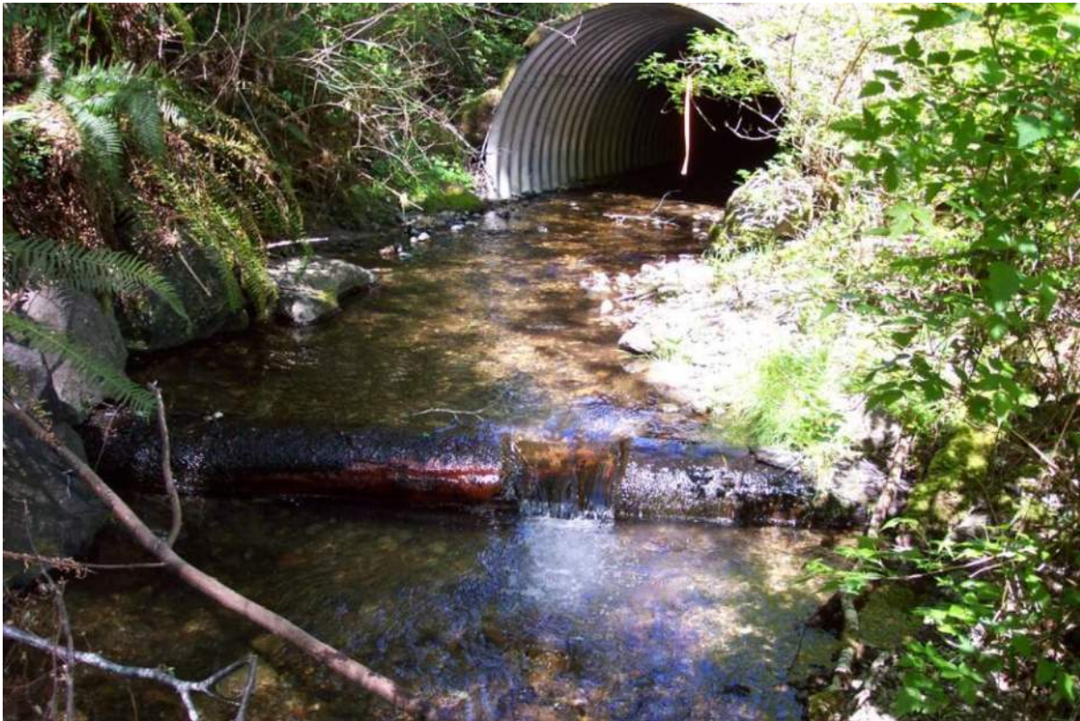
Figure 7.7: Log control used to control grade at the outlet of a culvert.
