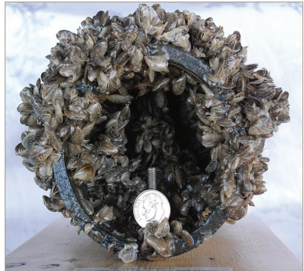
Quagga mussels encrust a pipe after three months’ growth.
