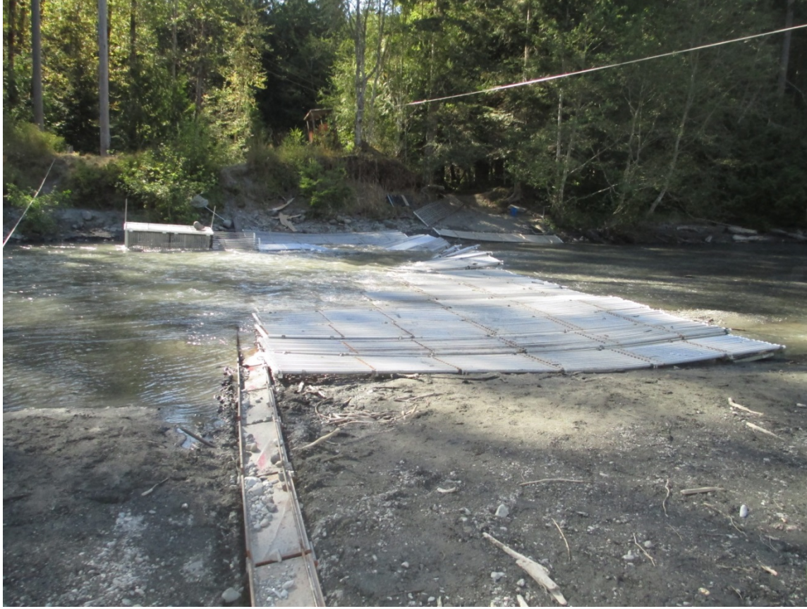
Figure 2. Link substrate rail system, visible in the foreground, with attached weir panels. Photo taken Aug 7, 2013, discharge = 760 cfs (USGS gage 12045500). Photo taken from central gravel bar looking back toward left bank channel.
