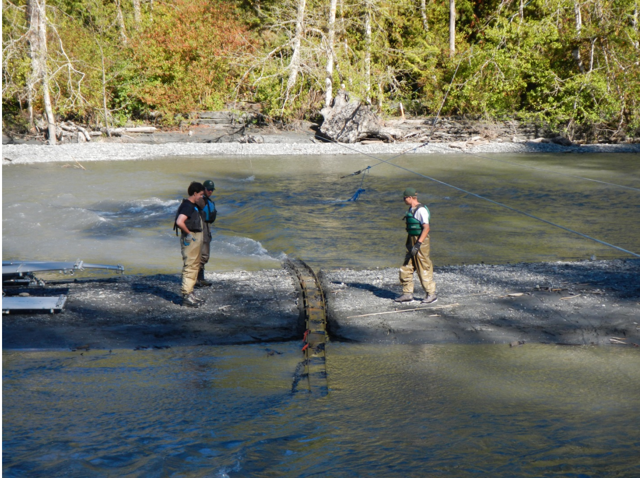
Figure 1. Newly designed, channel conforming substrate rail exposed on central gravel bar, looking from left bank channel across to right bank channel. Photo taken July 24 2013, discharge = 1,050 cfs (USGS gage 12045500).
