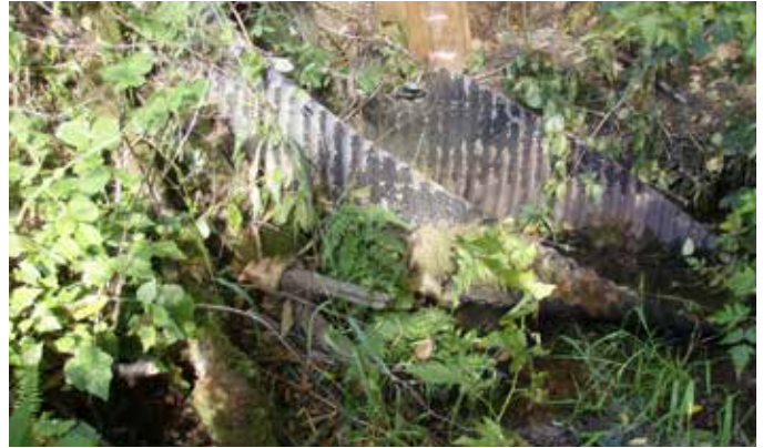
Failed culvert in Cedar Creek
