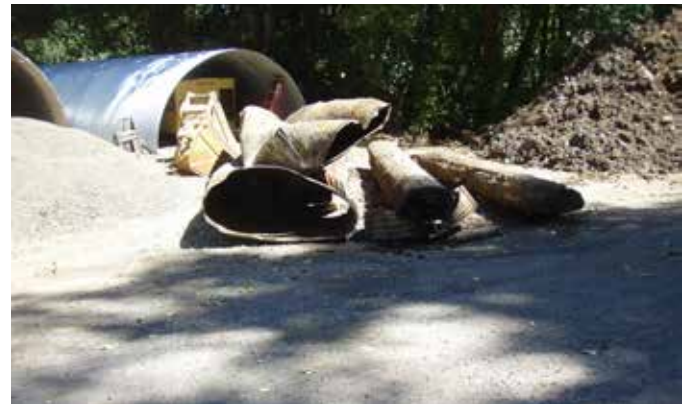
Failed culvert removed
