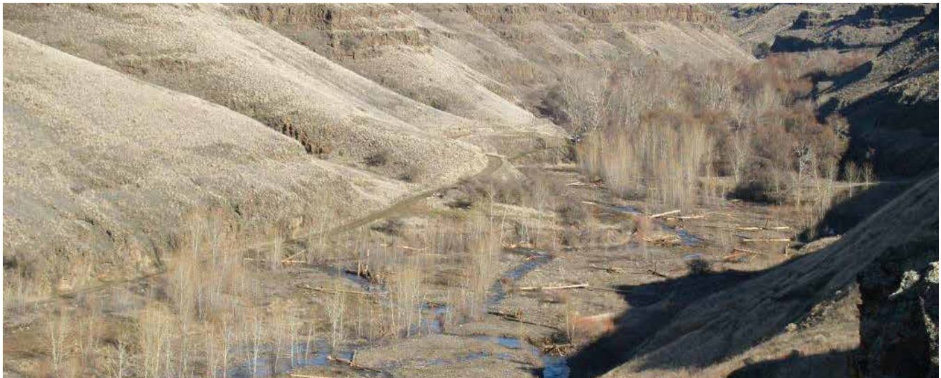
George Creek Restoration: Over 300 logs were used to create 70 large wood structures on 0.7 mile of George Creek. Floodplain function and instream habitat are improved in this Asotin County project.
