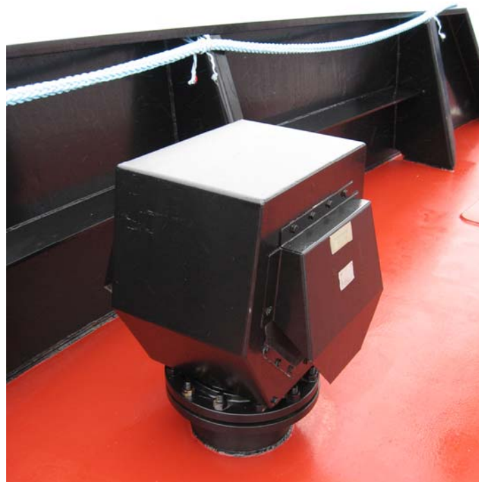
Figure A-3. Ballast tank vent.
