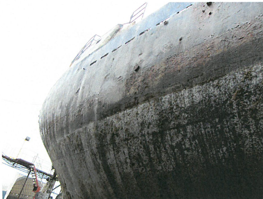
Figure 15 – Ecology photograph showing the starboard-side diver-plugged overboard discharge of the Deep Sea in drydock at Stabbert. Note the overboard is close to the waterline.
