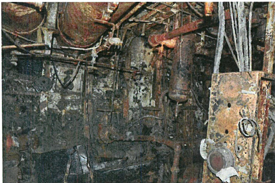
Figure 11 - King County Sheriff's Office investigator's photograph showing some of the damage to the engine room.
