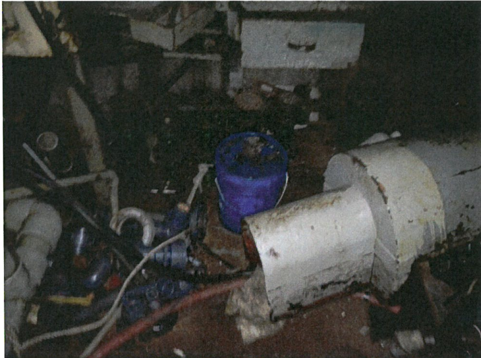
Figure 10 - USCG photograph from January 6, 2012, of the Deep Sea's engine room showing PVC piping pieces in no short supply.
