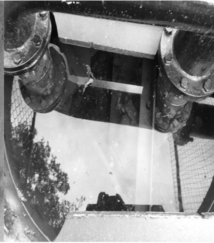
Water Supply Valve Pond #1
