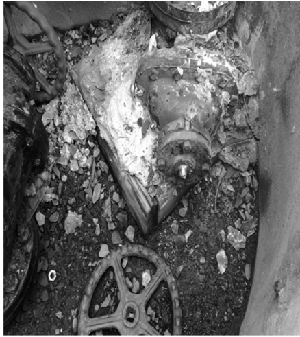
Water Supply Valve Pond #5
